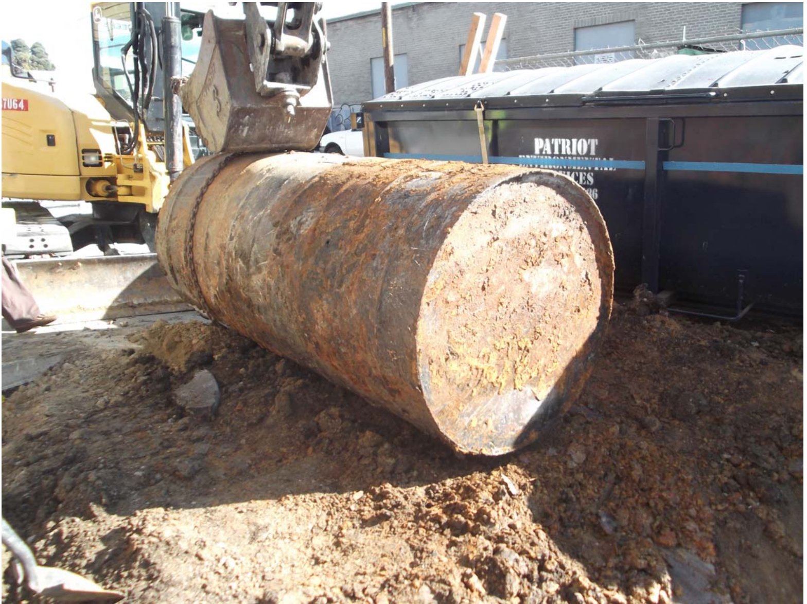
Image #2 Hole on north side in upper half on west half of UST.
