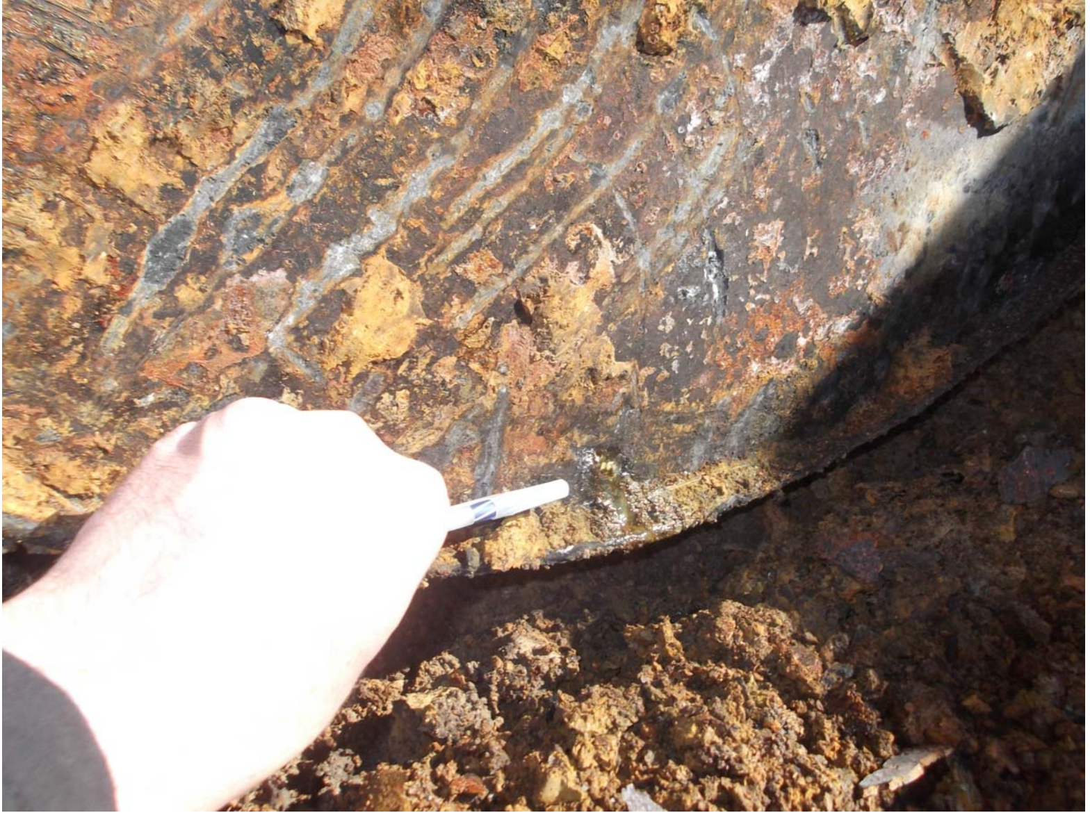
Image #4 Hole near bottom at west end of UST.
