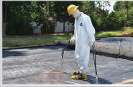
Geo-Seal CORE is spray applied to increase the systems tensile strength and provide a seamless membrane
