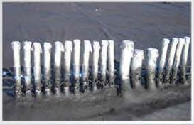
Penetrations are sealed individually
