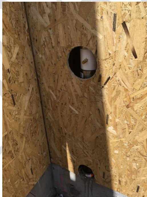
Photograph 2 – Riser Sampling Port at Exterior Wall at Ground Level (typical).
