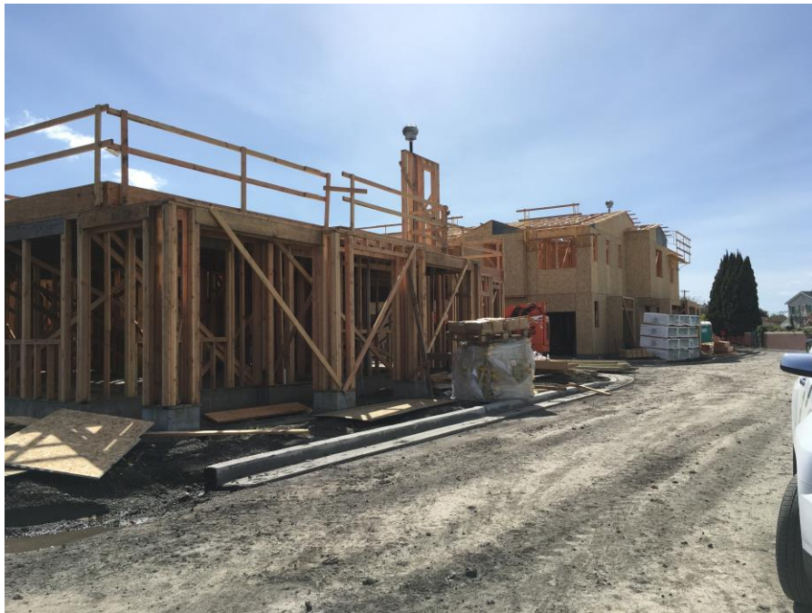
Photograph 1 – View of The Bungalows Buildings 1 through 4 with Wind Turbines installed at Roof Level.
