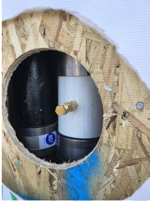
Photograph 3 – Riser Sampling Port at Exterior Wall at Ground Level (typical).
