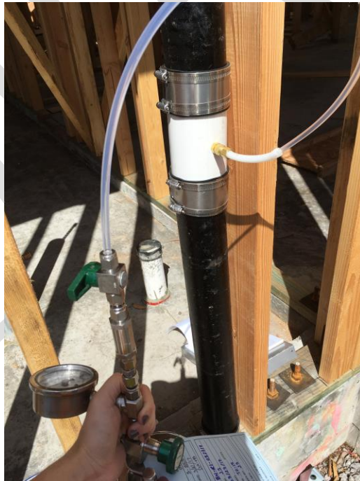
Photograph 4 –Riser Air Sample Being Collected into 1-Liter Summa Canister (typical).
