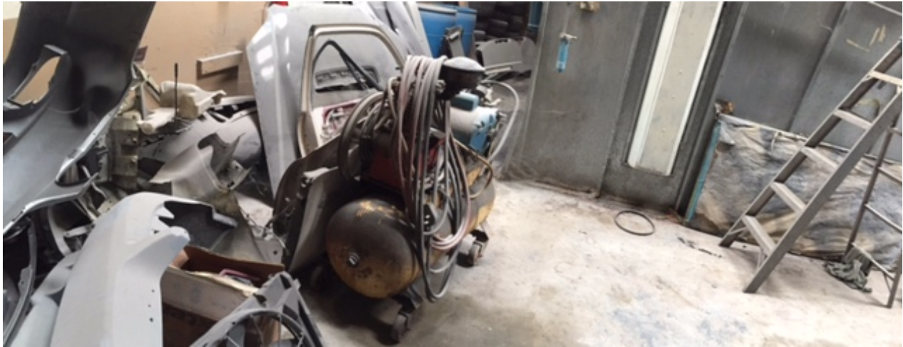
Photo 6: Subject Site (Facing North) One-Story Commercial Garage Building (Paint Booth in West Warehouse Area of A&C Auto Body & Frame Unit A)
