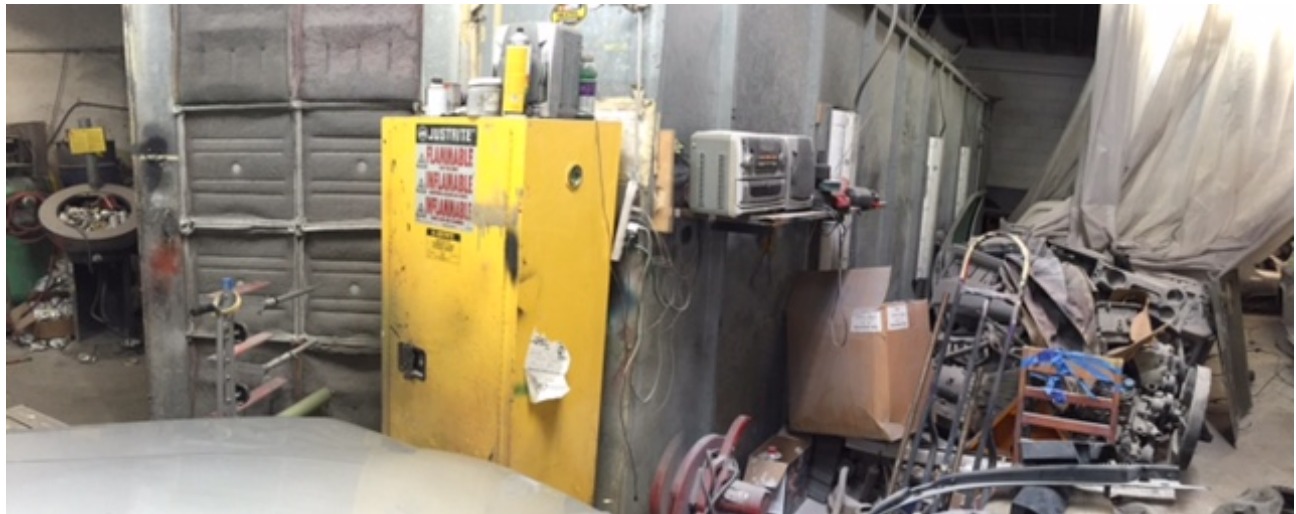
Photo 11: Subject Site (Facing Southwest) One-Story Commercial Garage Building (Paint Booth in Warehouse Area of JP Auto Body & Paint Unit C)
