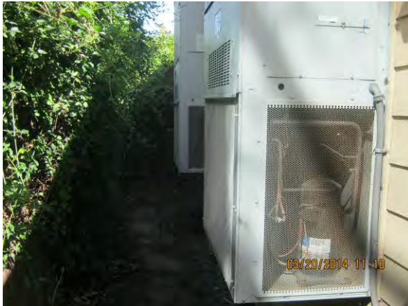
View along the western end of the 5219 Dover Street (CHRCO Sport Medicine Center) building showing the facility's HVAC equipment
