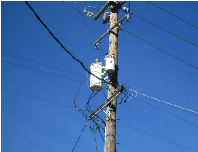
25. View of two pole-mounted transformers
