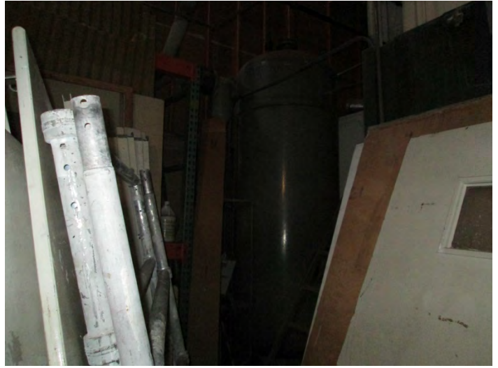
18. View of the hot water boiler tank
