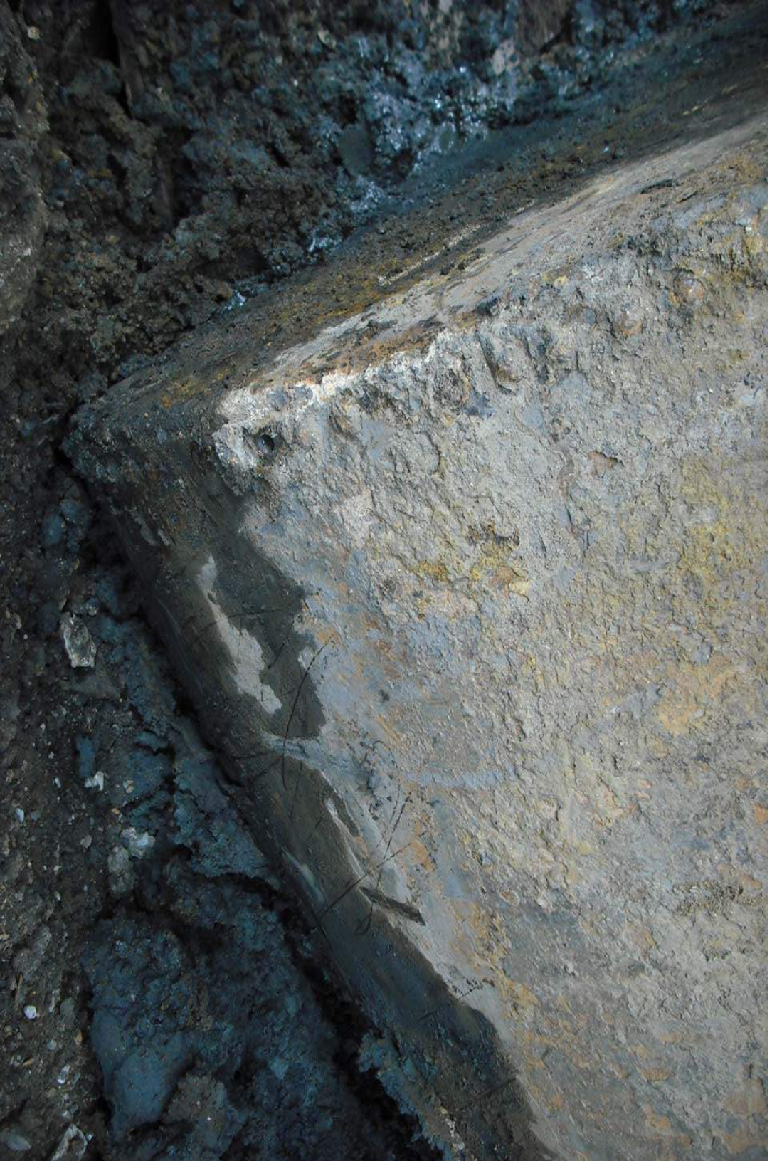
Missing rivet from UST
