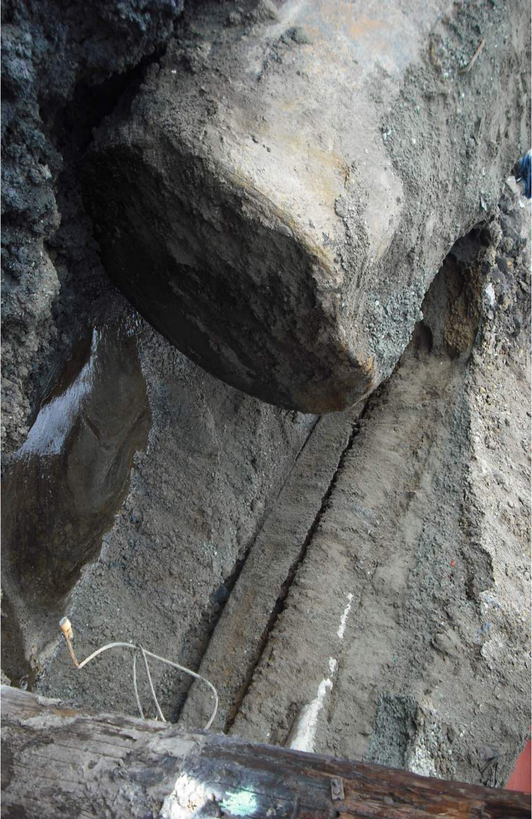
Oily water in UST pit
