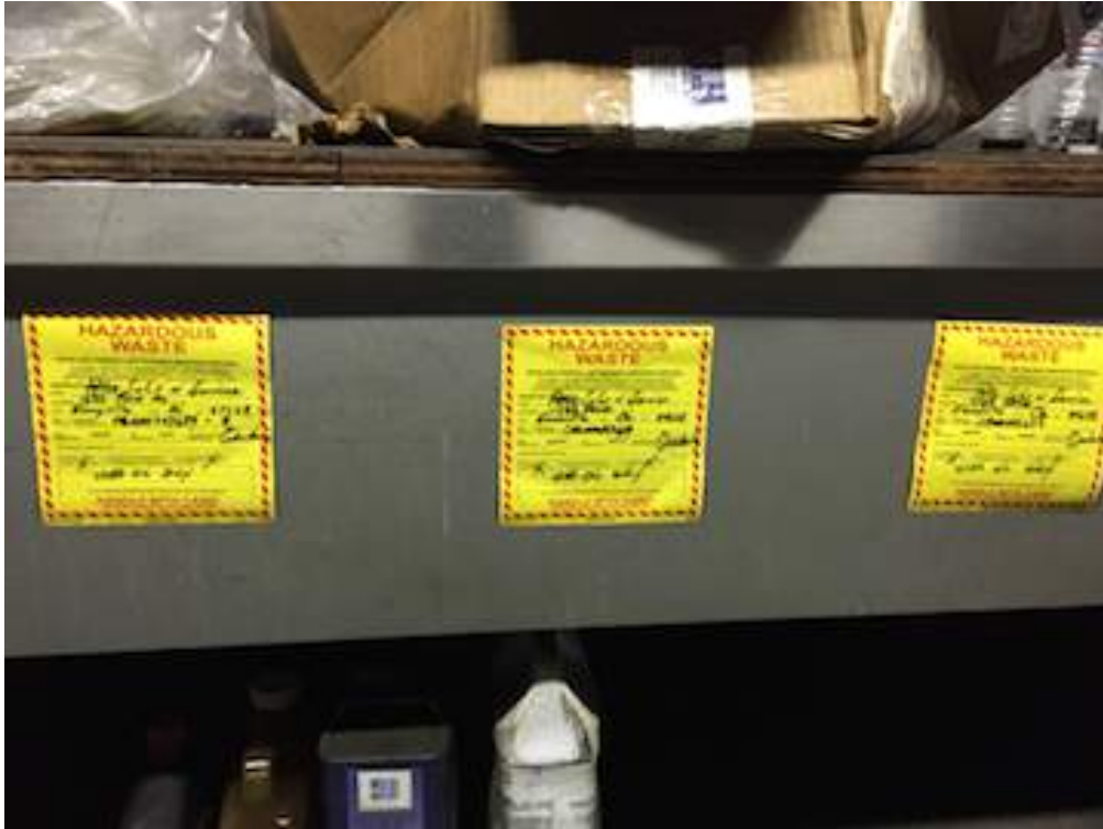
Photograph 7 – Used oil storage tank in corrugate metal building.
