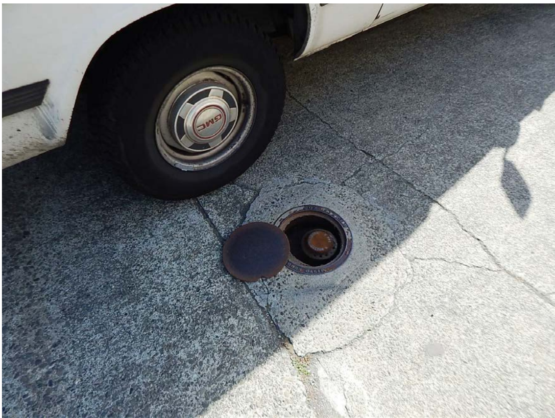
Photograph 5 - View of a fill port with the lid removed
