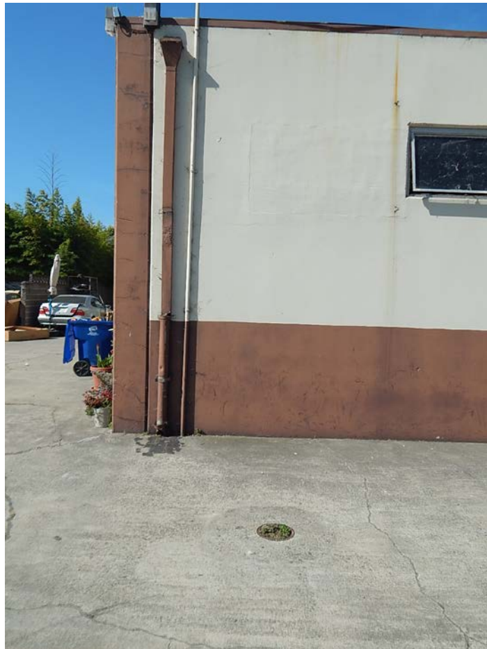
Photograph 4 - View of one of the UST fill ports and vent pipe
