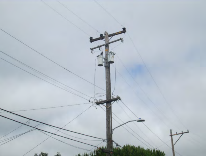
49. View of two pole-mounted transformers
