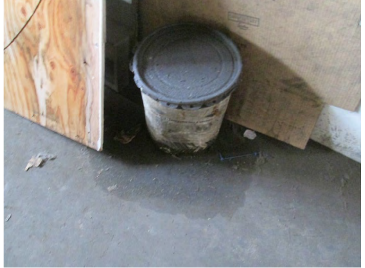
34. An unidentified substance container with staining; located on the third level
