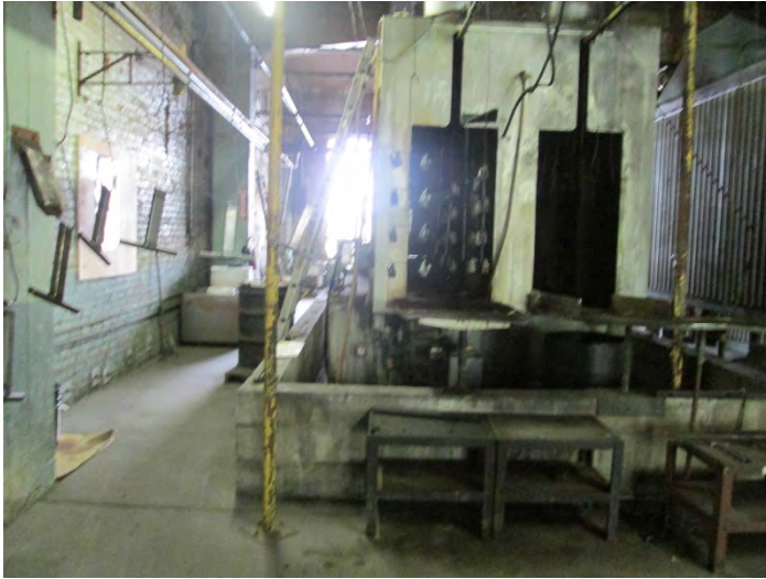
29. View of furnaces located in the third level of the warehouse
