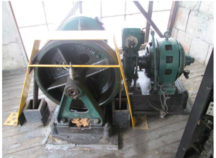
36. Elevator equipment located on the fourth level
