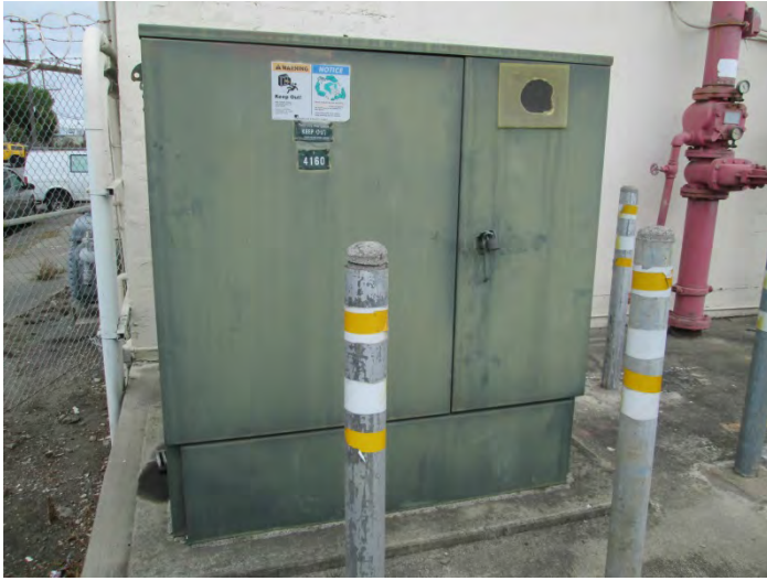
41. Pad-mounted transformer #2 located on the east side of subject property
