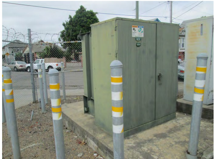
40. Pad-mounted transformer #1 located on the east side of subject property
