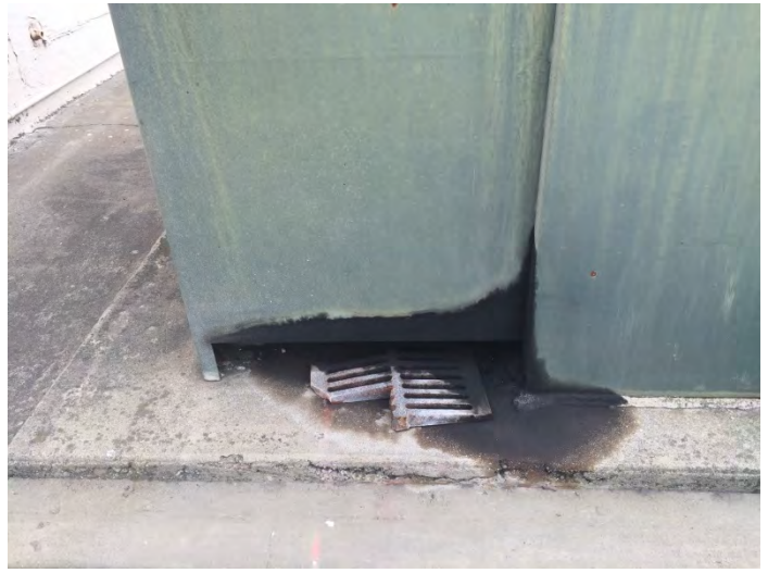
42. Staining found below pad-mounted transformer #2
