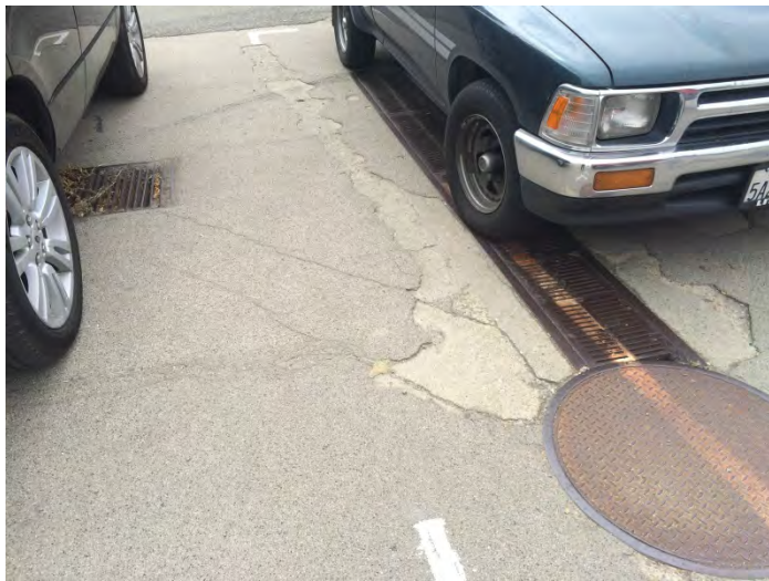
43. Two additional drains located on the east side of the subject property
