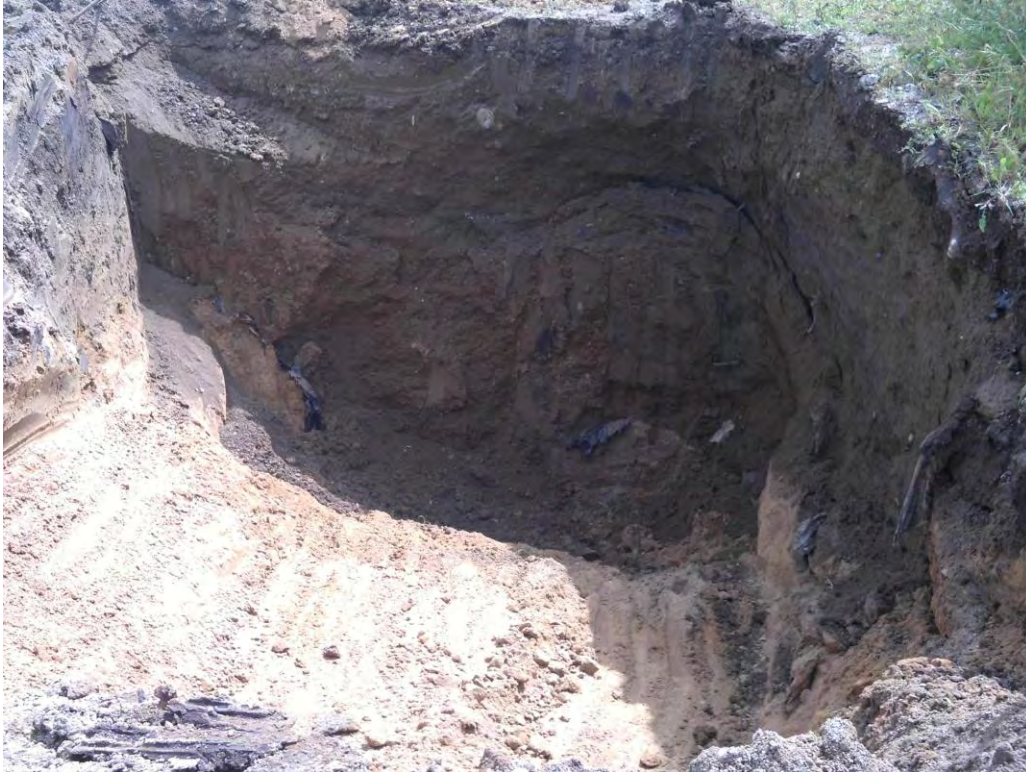
Photograph 3: Facing east at excavation, former import fill against east and south excavation wall.
