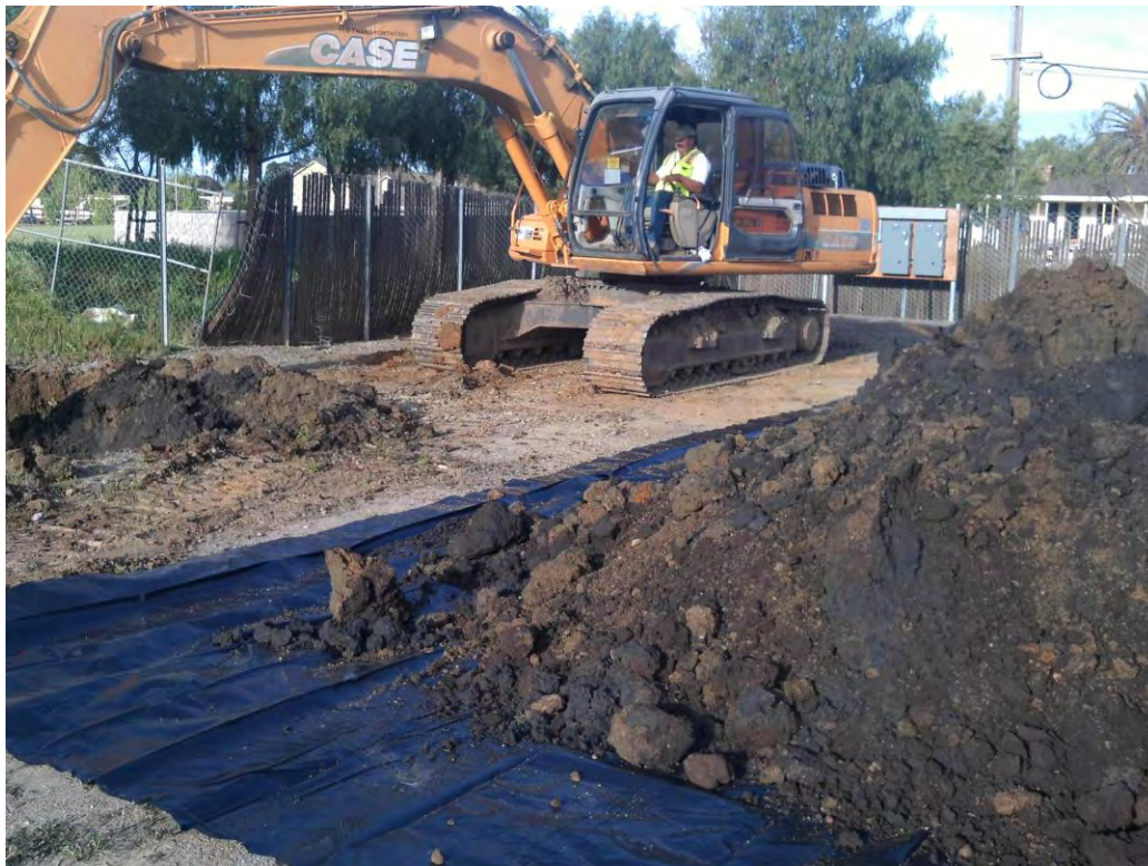
Photograph 2: Final excavation activities to remove oil impacted soils in former power pole vicinity.
