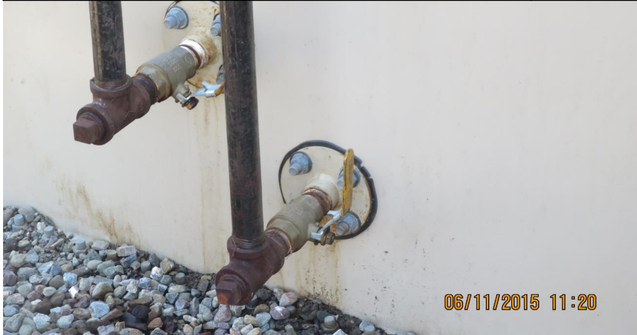
DESCRIPTION: STOCK TANK #1 – VALVES WIL MINOR WEEPING. Photo # 18 of 26
