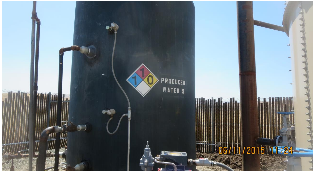
DESCRIPTION: POLISHER WATER TANK Photo # 19 of 26
