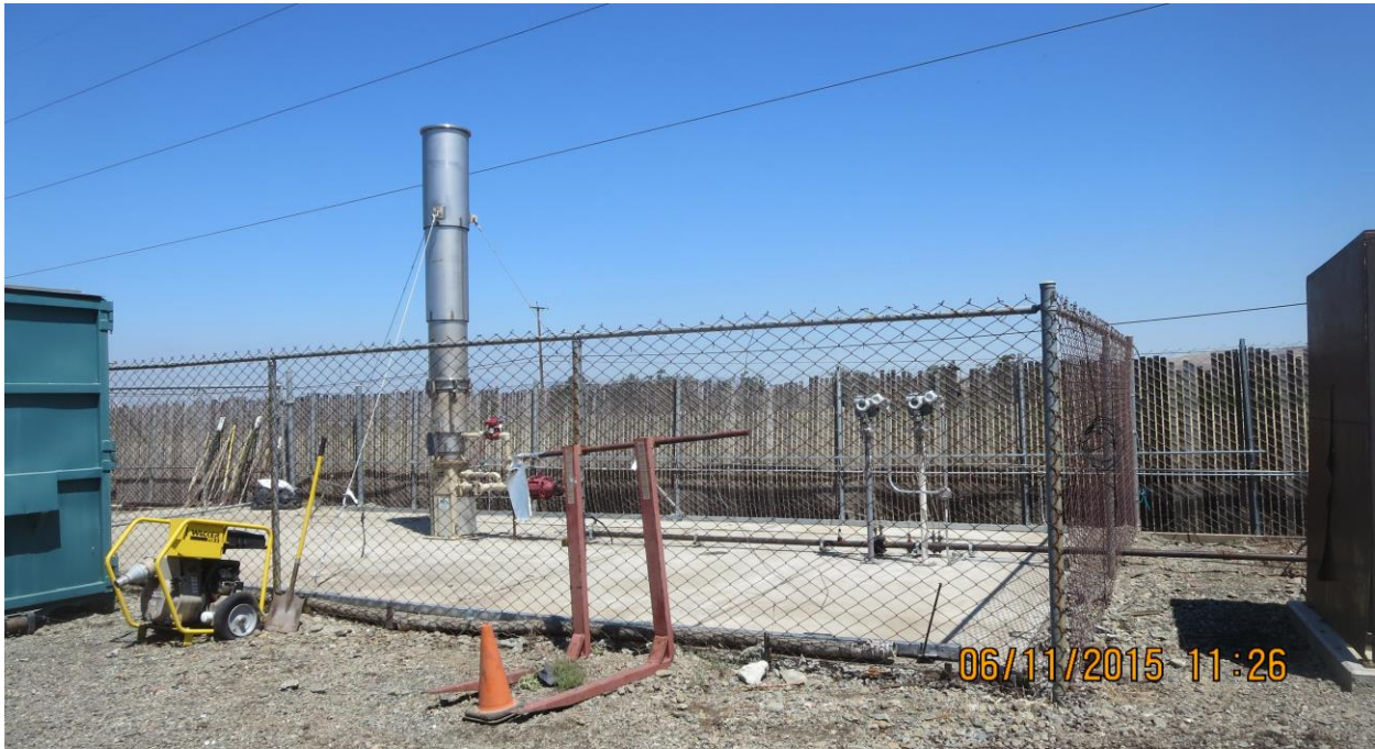
DESCRIPTION: ENCLOSED COMBUSTION SYSTEM
