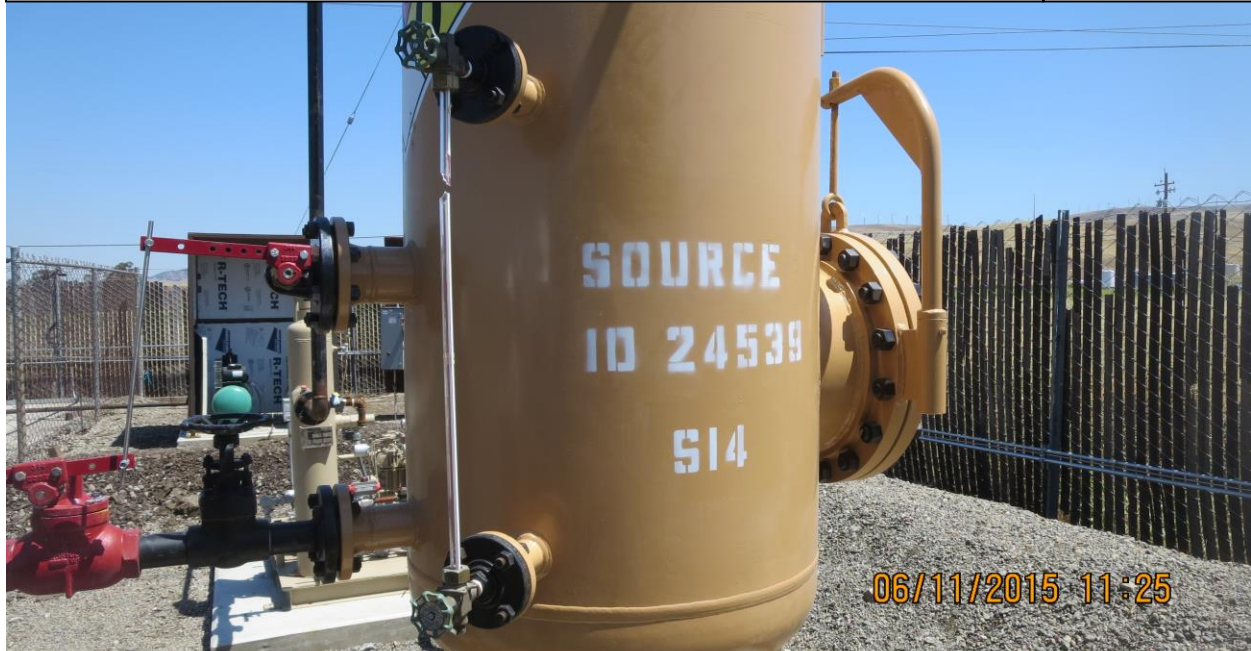
DESCRIPTION: CURRENTLY CLOSED SYSTEM, LEVEL GAUGE IS BROKEN Photo # 20 of 26
