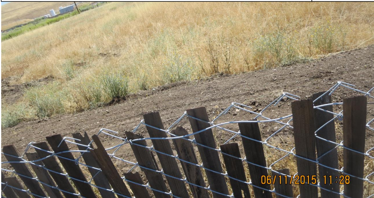
DESCRIPTION: SOIL BERM OUTSIDE THE FENCE BETWEEN FACILITY AND CREEK
