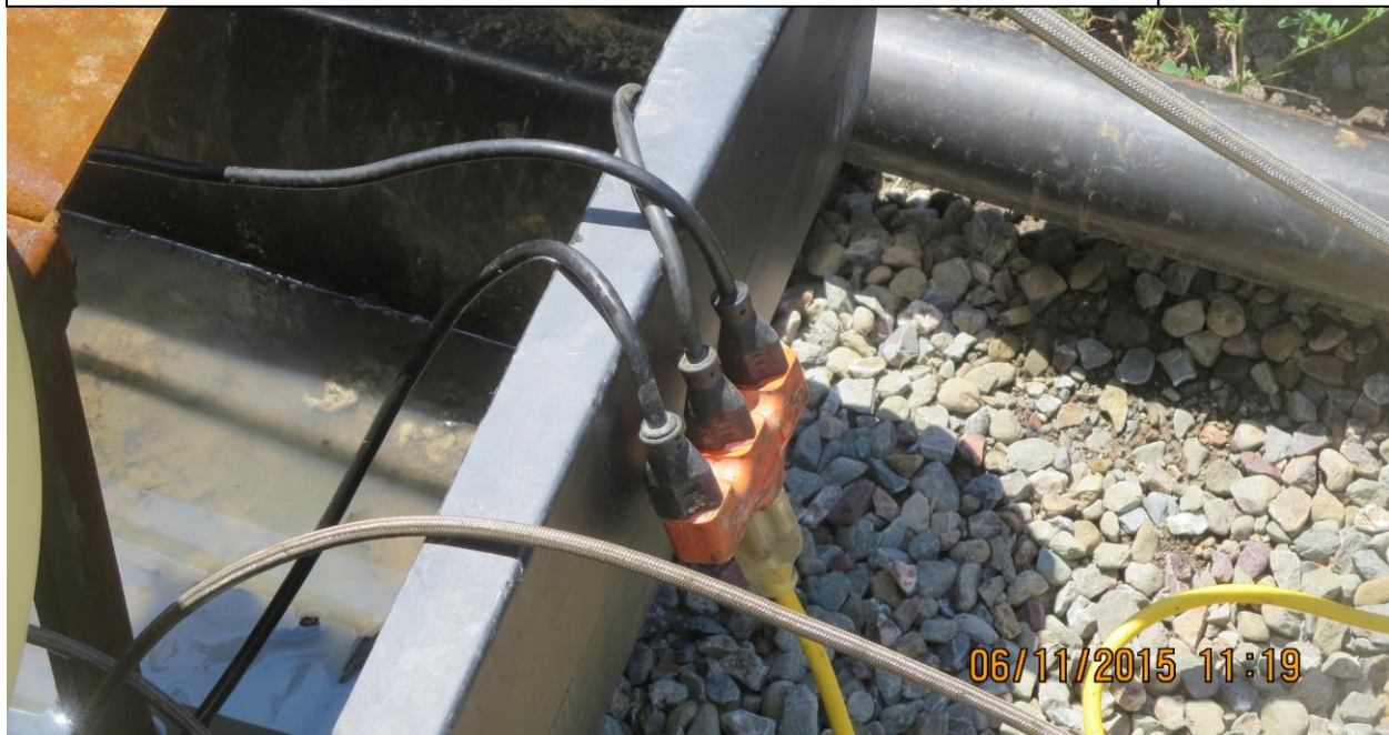
DESCRIPTION: SCORTRON MATERIALS WITH ELECTRICAL CORDS Photo # 16 of 26
