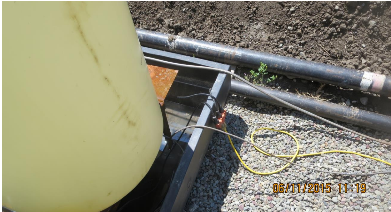
DESCRIPTION: SCORTRON MATERIALS WITH ELECTRICAL CORDS Photo # 15 of 26
