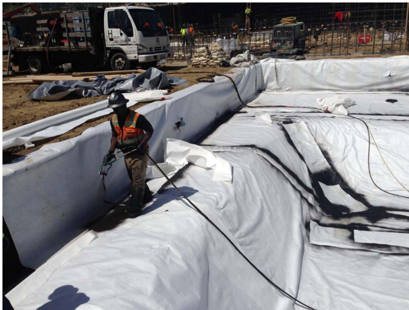
Photo 1. Installation of the Geo-Seal BOND Layer fabric on top of the cured Geo-Seal CORE Spray at the northeastern elevator pit footing of Building A. Photograph taken on April 14, 2017.
