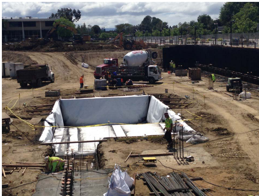
Photo 2. Installation of the Geo-Seal BOND Layer fabric on top of the cured Geo-Seal CORE Spray at the southwestern elevator pit footing of Building A. Photograph taken on April 12, 2017.
