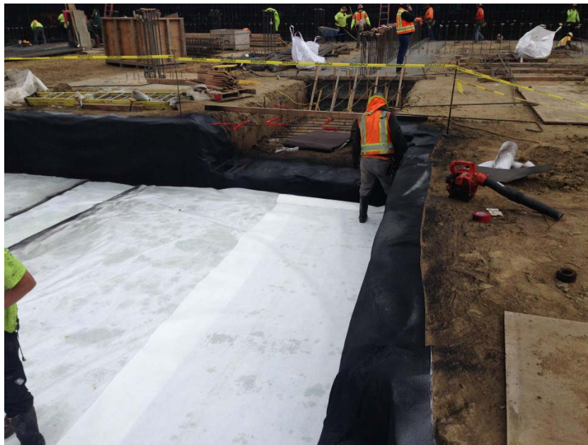
Photo 1. Typical termination of the vapor barrier fabric, extending one foot or more beyond the edge of the elevator pit footing. Installation of the Geo-Seal BOND Layer fabric on top of the cured Geo-Seal CORE Spray at the southwestern elevator pit footing of Building A. Photograph taken on April 12, 2017.
