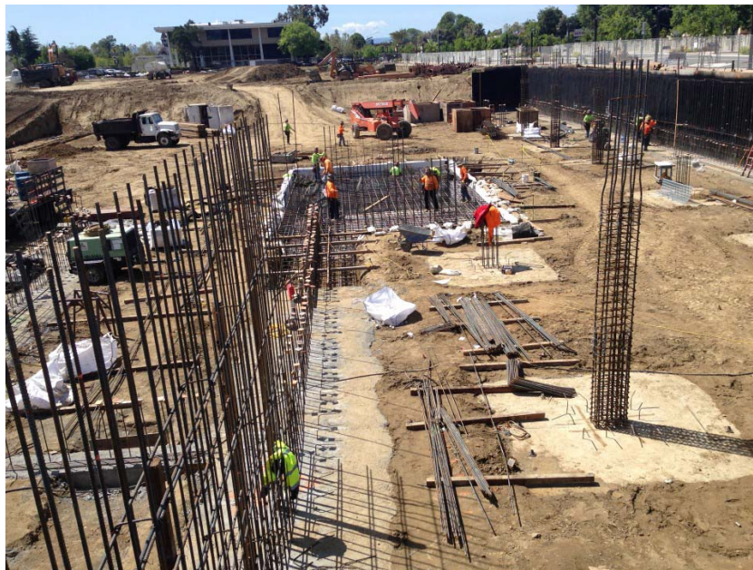
Photo 1. Installation of rebar at the southwestern elevator pit footing of Building A during follow up inspection to check for any penetrations. Photograph taken on April 14, 2017.
