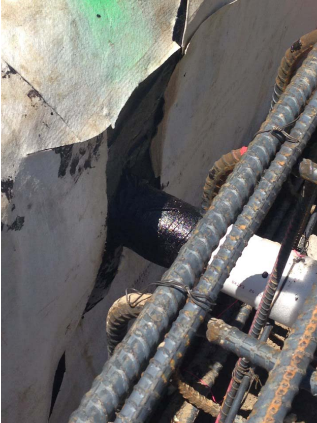
Photo 1. Repair of a plumbing penetration of the vapor barrier at the northeastern elevator pit footing of Building A. Photograph taken on April 21, 2017.
