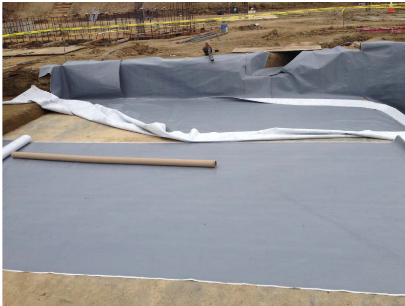
Photo 2. Beginning of the installation of the Geo-Seal BASE Layer fabric at the southwestern elevator pit footing of Building A. Photograph taken on April 11, 2017
