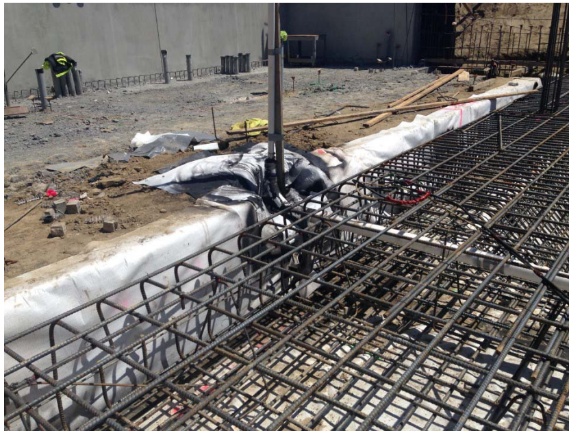
Photo 2. Repair and addition to the vapor barrier at a plumbing penetration at the northeastern elevator pit footing of Building A. Photograph taken on April 21, 2017.
