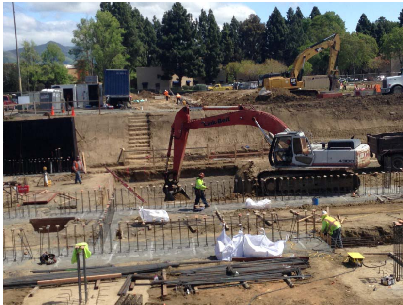
Photo 2. Excavation of the northeastern elevator pit footing area of Building A prior to the placement of the Geo-Seal BASE Layer fabric. Photograph taken on April 12, 2017.
