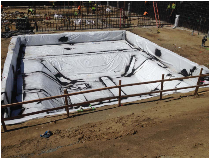
Photo 2. Installation of the Geo-Seal BOND Layer fabric on top of the cured Geo-Seal CORE Spray at the northeastern elevator pit footing of Building A. Photograph taken on April 14, 2017.
