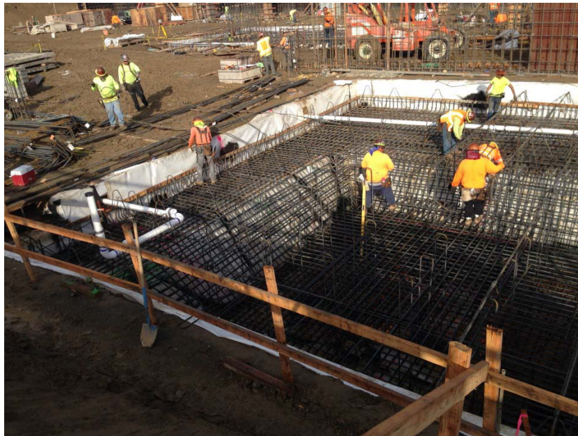
Photo 2. Installation of rebar at the northeastern elevator pit footing of Building A during follow up inspection to check for any penetrations. Two plumbing penetrations can be seen at the upper left of the photograph. Photograph taken on April 20, 2017.
