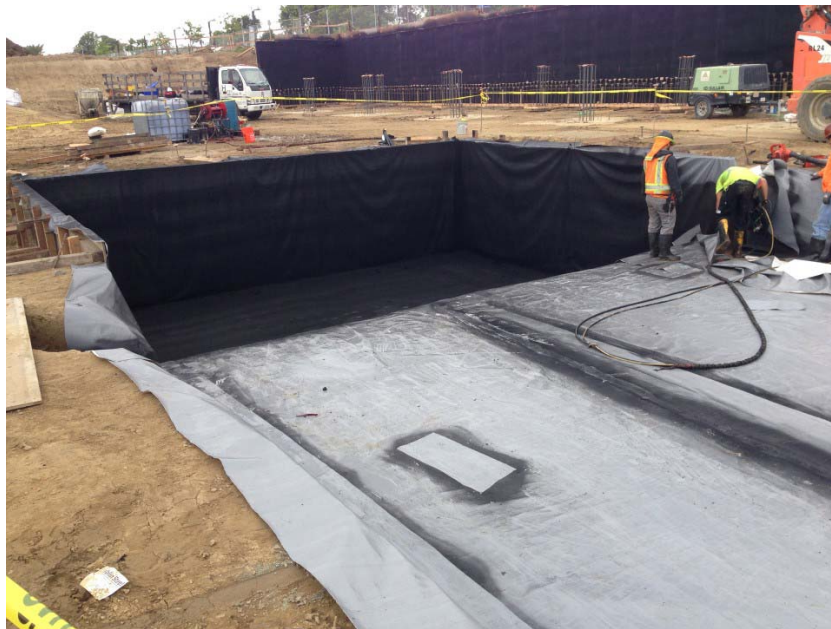
Photo 1. Installation of the Geo-Seal BASE Layer fabric and spray application of the Geo-Seal CORE Spray at the southwestern elevator pit footing of Building A. Photograph taken on April 12, 2017.
