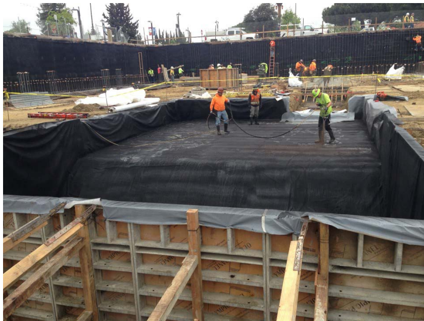
Photo 2. Spray application of the Geo-Seal CORE Spray at the southwestern elevator pit footing of Building A. Photograph taken on April 10, 2017. Photograph taken on April 12, 2017.
