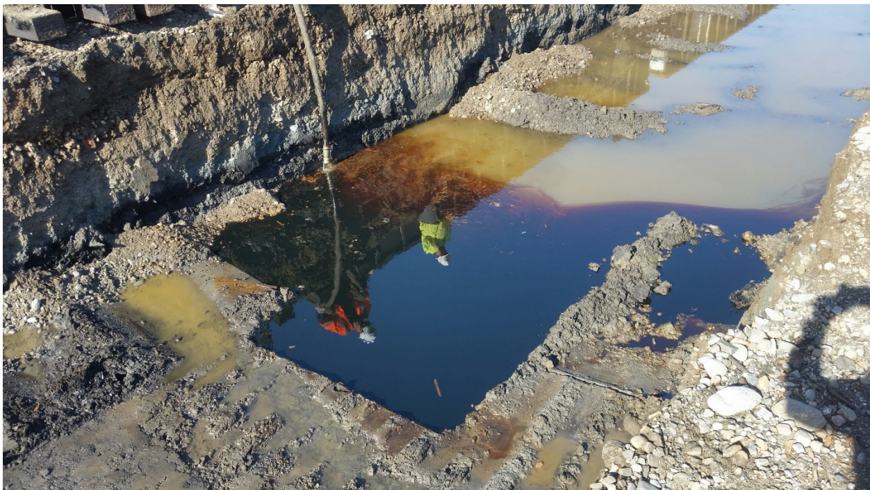
04.10.2015 Product and water in the excavation. This liquid was removed and product was not visible in the excavation at the completion of the excavation activities.
