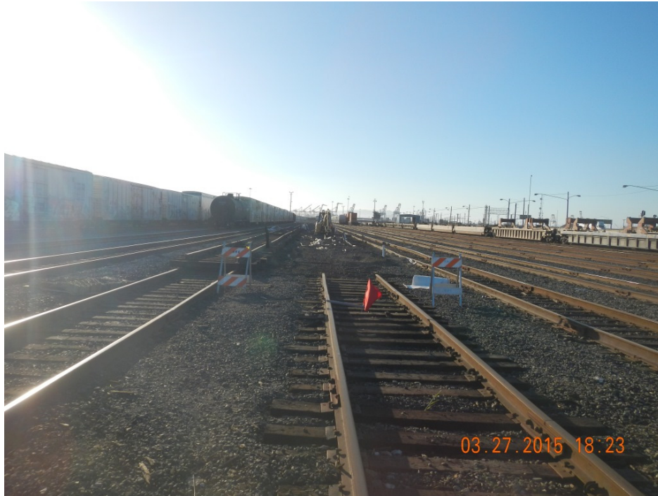
03.27.2015 Trench #1 and Trench #2 excavation completed, PVC piping installed, and trenches backfilled with native soil.
