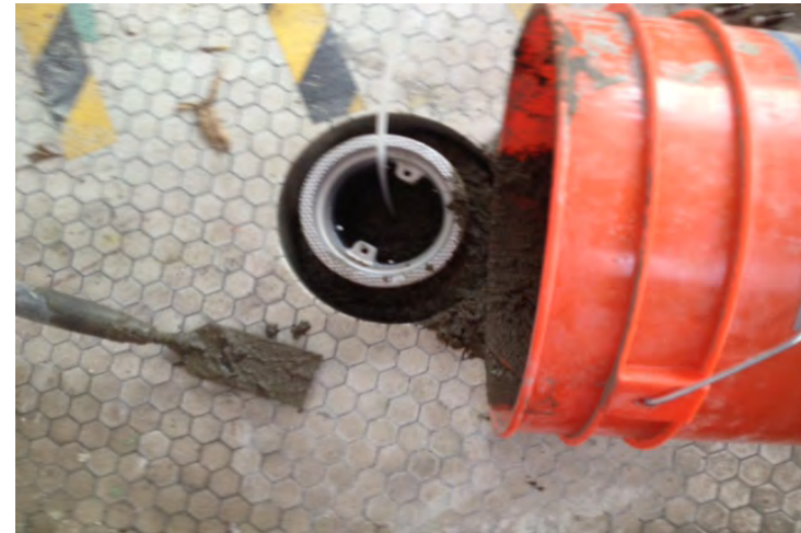
Vapor Monitoring Well Completion, Indoors
