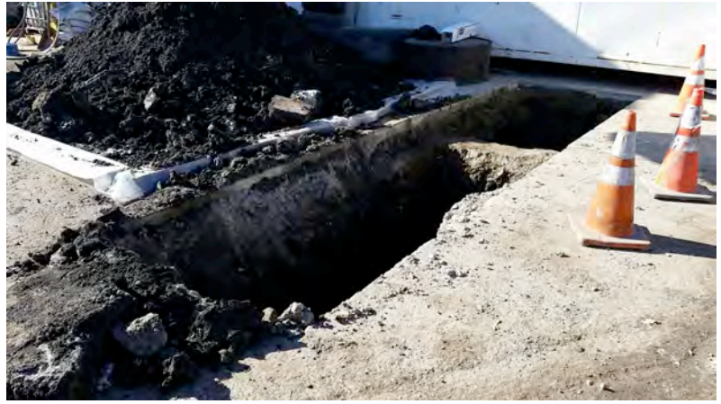
View of excavation looking to the southwest. Note concrete conduit in the western 1/3 of the excavation.
