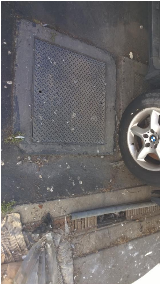
INACTIVE OIL WATER SEPARATOR
