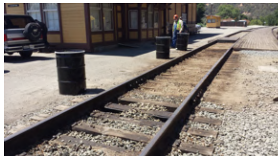
VIEW OF EXCAVATED TRACKS LOOKING SOUTHWEST. NOTE THREE OF FOUR FILLED SOIL DRUMS PRESENT ADJACENT TO EXCAVATED TRACKS AREA.
