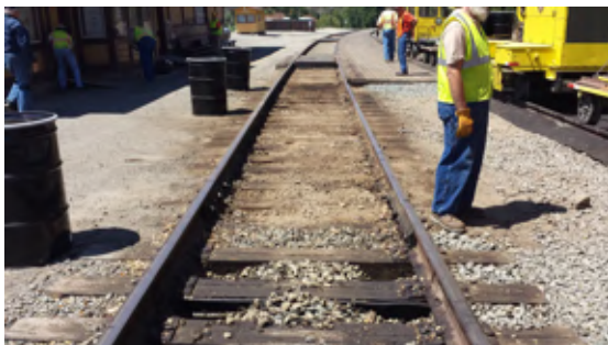
VIEW OF EXCAVATED TRACKS LOOKING WEST. BALLAST-ONLY AREA IS ON LOWER SIDE OF PHOTO, AND DIRT BALLAST AREA IS ON MIDDLE AND UPPER SIDE OF PHOTO.
