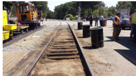
VIEW OF COMPLETED EXCAVATION, LOOKING EAST. SUNOL DEPOT IS ON FAR RIGHT EDGE OF PHOTO.
