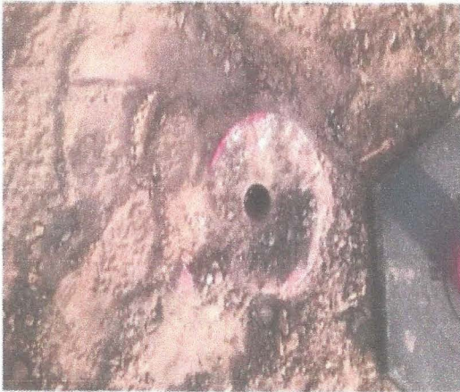
Damaged Monitoring Well MW-2
