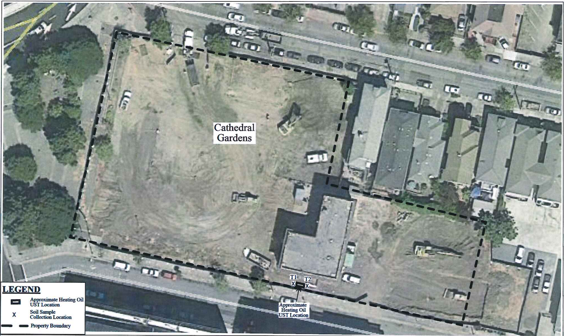
Figure 2 Site Plan Aerial Photograph Showing Approximate UST Location Cathedral Gardens 638 21st Street Oakland, California
