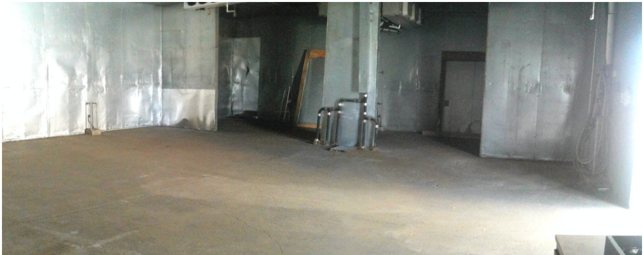
Photo 12: Subject Site (Facing Southeast) Building 3 (Cold Storage Building) Former Cold Storage Rooms
