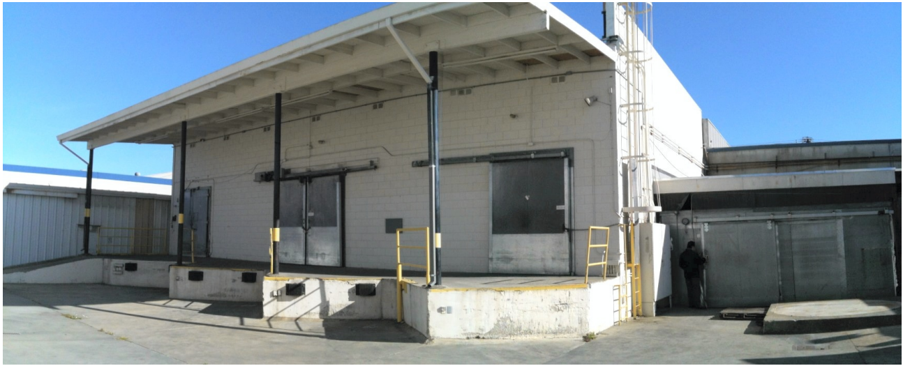
Photo 11: Subject Site (Facing North) Building 3 (Cold Storage Building) Former Cold Storage Rooms
