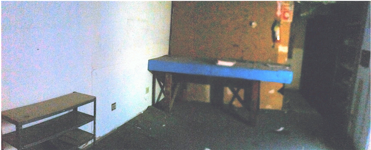
Photo 15: Subject Site (Facing North) Building 4 (Dry Goods Storage Building) Northeast Storage Room
