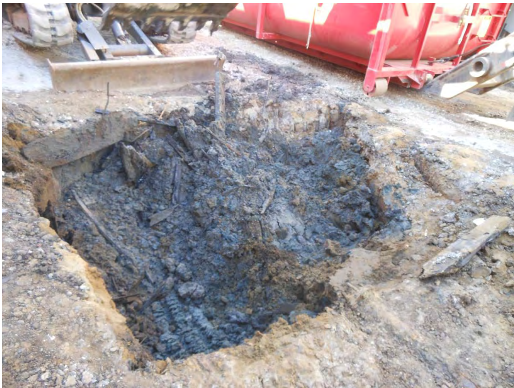
Photo 2 Redwood Debris and Contaminated Soil
