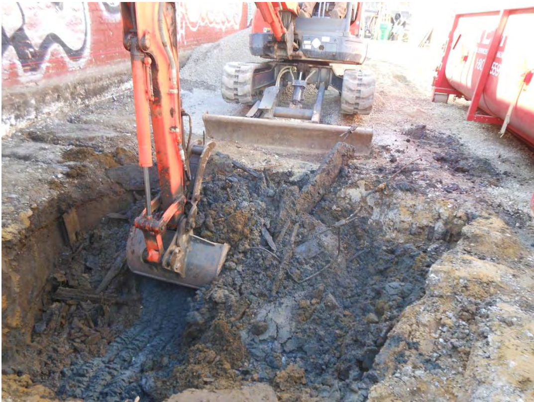
Photo 1. Top of Redwood UST Encountered, Note Gray Contaminated Soil
