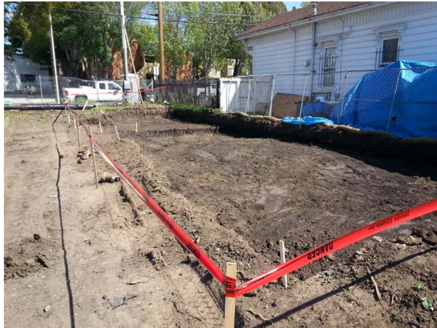
Photograph 11: The completed remedial excavation on the south side of the former 16331 Kent Avenue site building.
