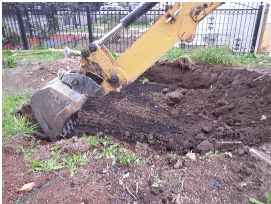
Photograph 6: Performing remedial excavation at the south side of the former 16331 Kent Avenue site building.
