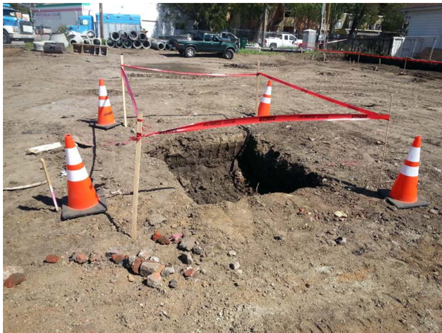
Photograph 10: The completed remedial excavation at boring L10 on the northwest side of the former 16331 Kent Avenue site building.
