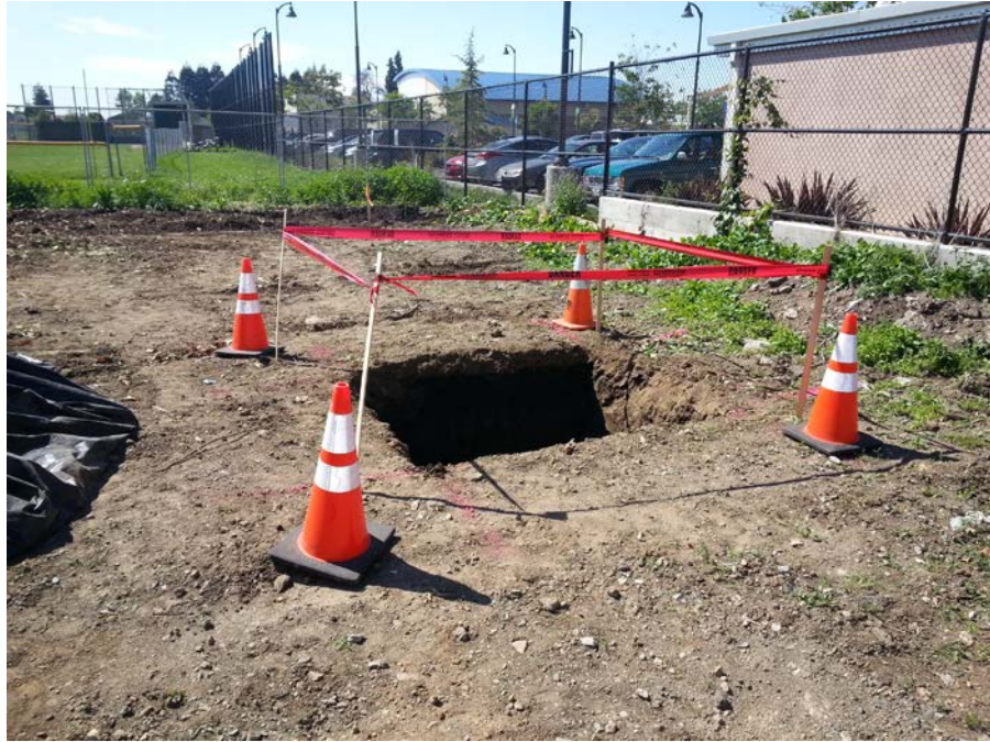
Photograph 9: The completed remedial excavation at boring CP3 in the former car port area of the site.
