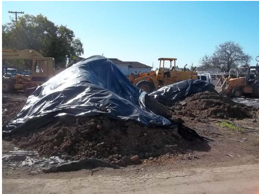
Photograph 5: Stockpiles stored on the site which were generated during trenching in Kent Avenue and East 14 th Street.
