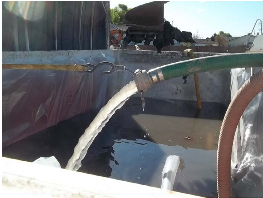
Photograph 3: Water pumped from the water cistern was stored in a plastic lined roll-off bin.
