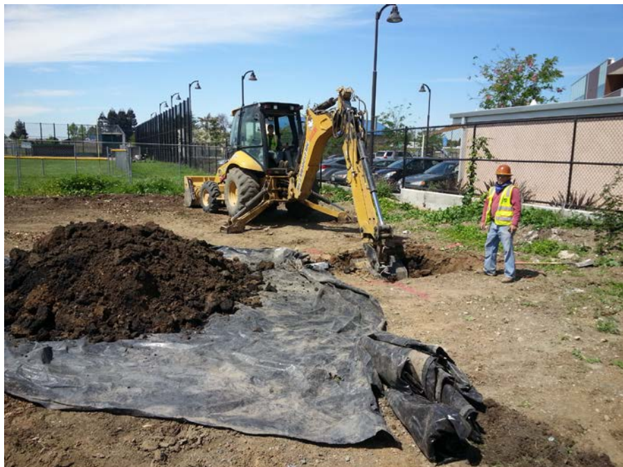
Photograph 8: Performing remedial excavation at boring CP3 in the former car port area of the site and temporary stockpile to be added to stockpile SP8.
