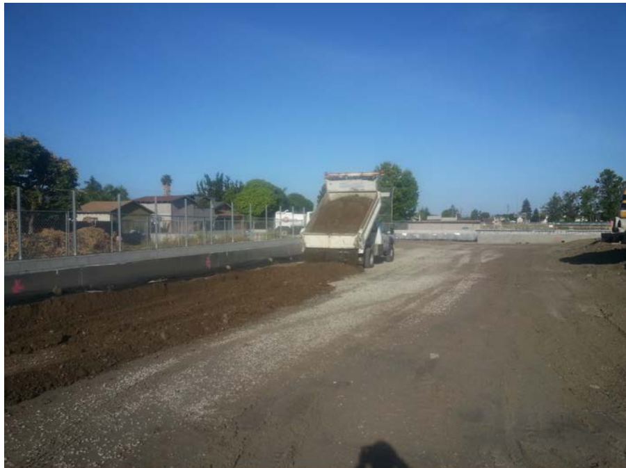
Photograph 14: Spreading soil for reuse from stockpile SPA on the southern portion of the site in an area designated to be paved and used as parking.
