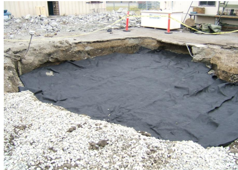
12. June 25, 2010 – Geotextile fabric has been laid to separate the sand from the drainage rock in the UST excavation.
