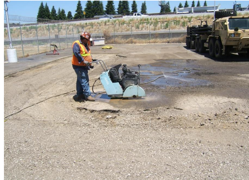
18. June 30, 2010 – Sawcutting clean lines in the old asphalt to prepare for the new asphalt.
