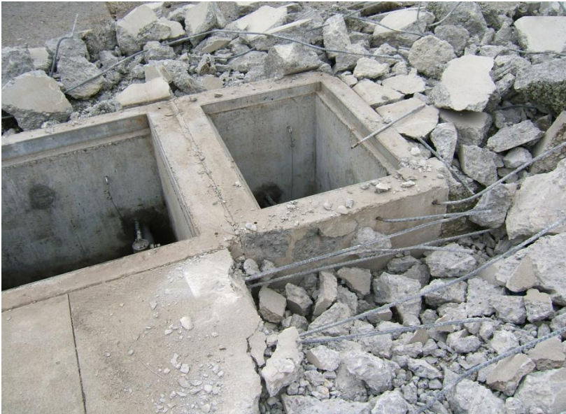
9. June 24, 2010 – Concrete and exposed rebar to be removed prior to the removal of the sump vaults.
