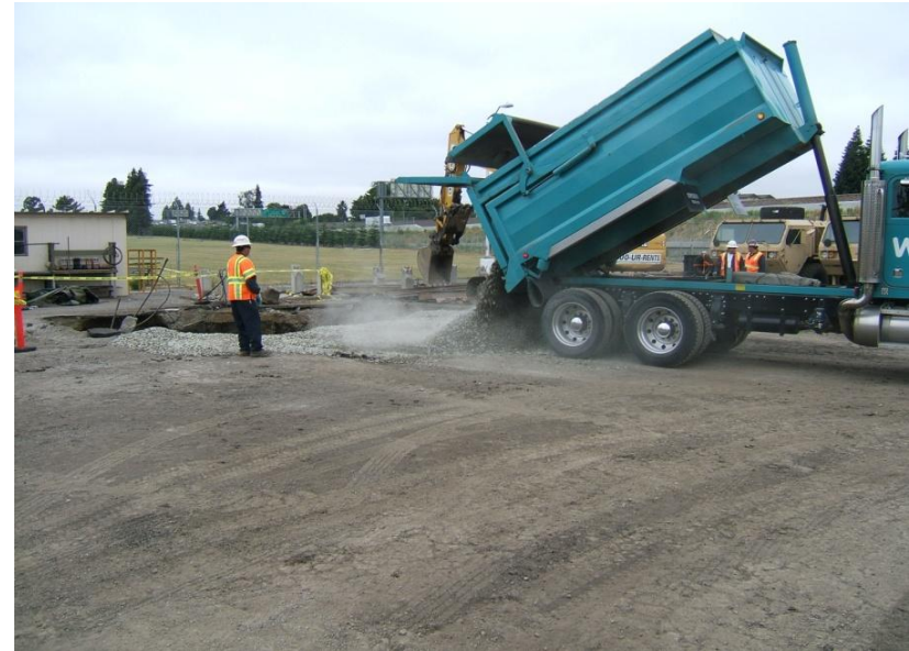
10. June 25, 2010 – The arrival of drainage rock to be placed within the excavations.
