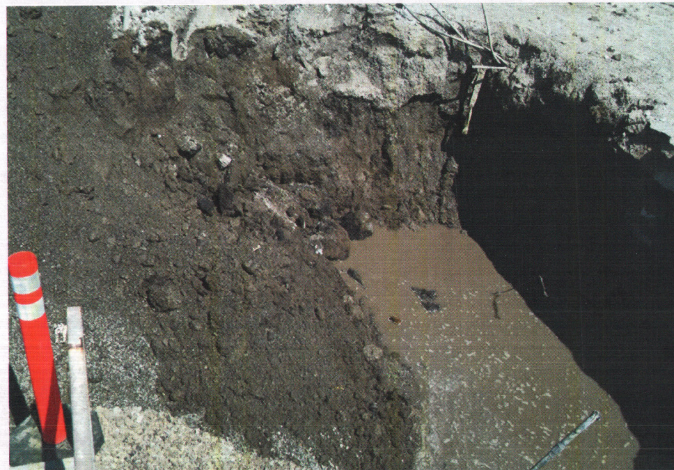
Pit sidewall collapse
