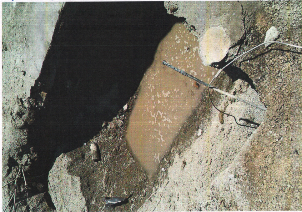
Groundwater infiltration into tank pit
