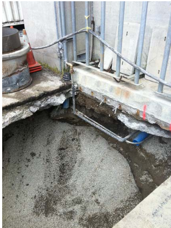
Photo 6 – View of excavation after UST and associated electrical and fuel lines had been removed up to building.
