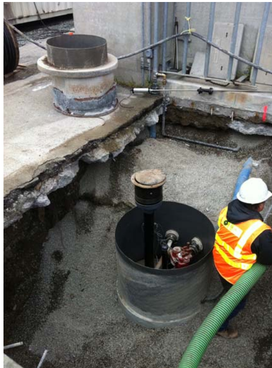
Photo 2 – View of UST excavation during removal of pea gravel using vacuum trailer.
