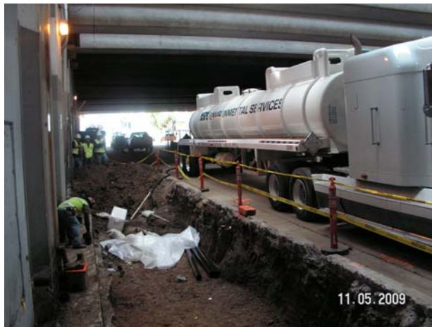
Photo 3 – View of product being pumped out of tank by NRC Environmental Services.
