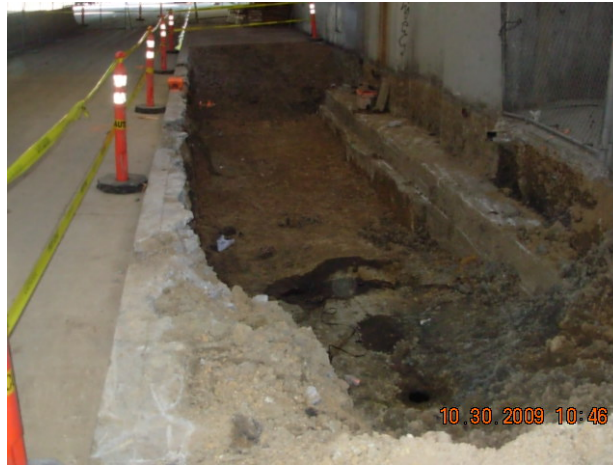
Photo 1 – View of top of UST. Top of UST has oily staining.
