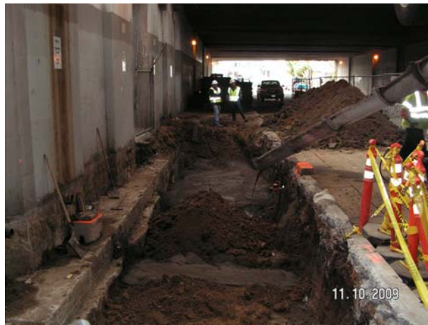
Photo 8 – View after excavation was nearly backfilled on 10/10/09. Three-foot wide can be seen backfilled in the foreground.
