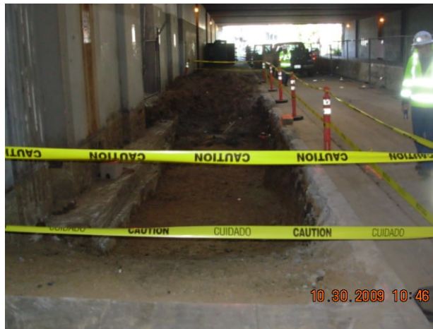
Photo 2 – View looking west down 29 th Street. UST is located on the other end of the excavation area.
