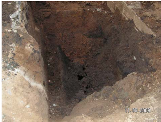
Photo 5 – View of product in bottom of excavation after the UST had been removed.
