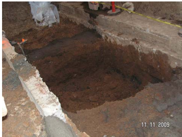
Photo 9 – View of excavation on 10/11/09 after additional soil was removed between excavated areas on 10/10/09.
