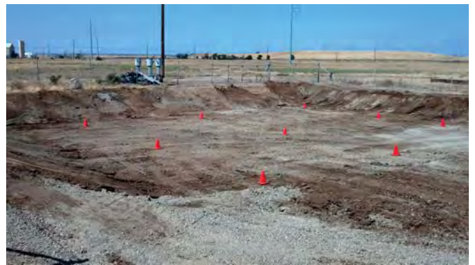
Photograph 6: Surface Impoundment Removed Exposing Native Soil. Cones Denote Soil Sample Locations (View to the northeast).
