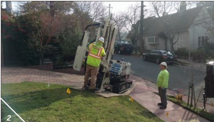
Photograph No. 3 – East view of residence front yard showing EnProbe personnel at Field Point B5, clearing borehole to 4 fbg to clear for unmarked subsurface utilities prior to using GeoProbe drilling equipment; approximate location of existing sanitary sewer service lateral shown as green dashed line (WGE, 1/17/18).
