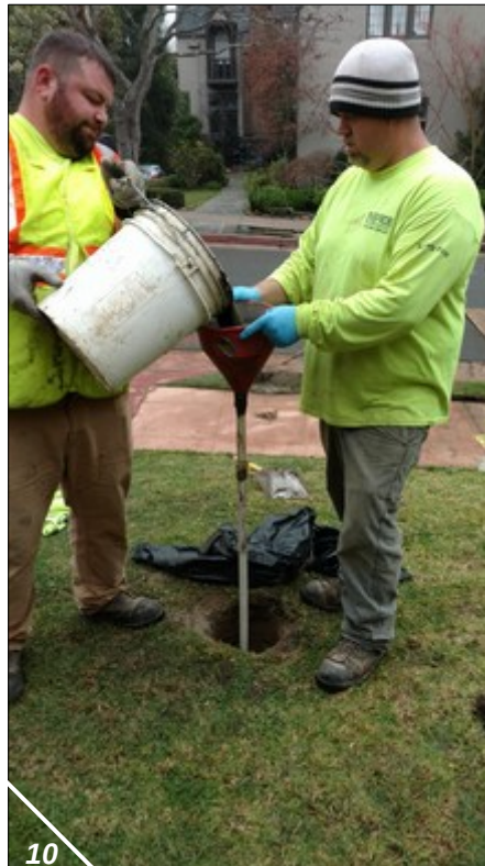
Photograph Nos. 10 & 11 – Views of EnProbe personnel during borehole backfilling activities; backfilling by tremie grout was requested by Alameda County Public Works Agency inspector at Field Point B5 due to small volume of drainage water observed in borehole on January 18, 2018 (WGE, 1/18/18).
