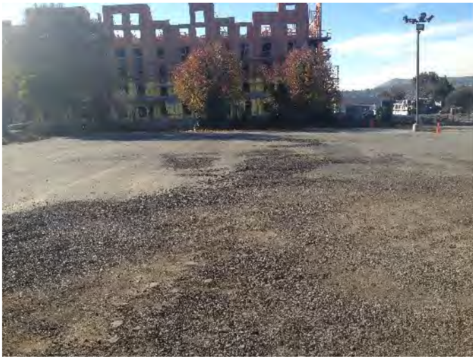
AN EXAMPLE OF THE CRACKED PAVEMENT AT THE SITE. TAKEN FROM THE MIDDLE OF THE SITE FACING WEST
