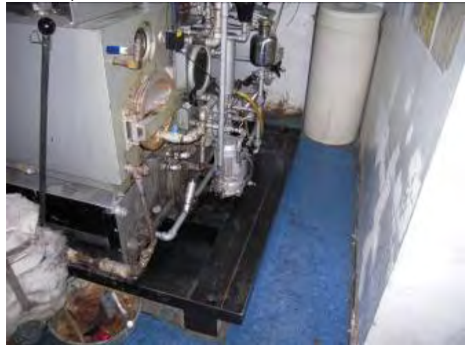
17. View of rear of PERC dry cleaning machine at the Site.
