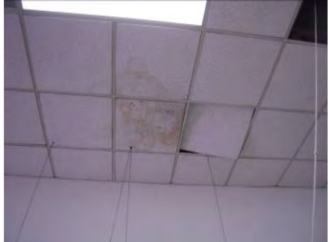
8. View of water damage inside packaging store tenant space.
