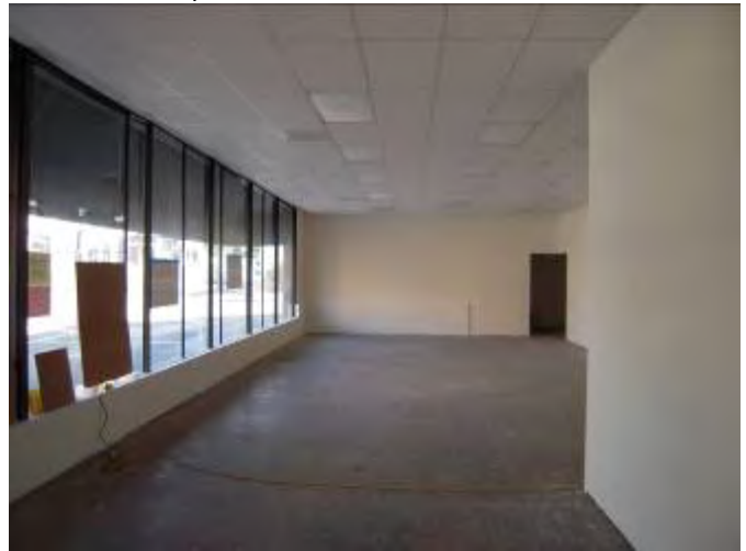
23. View of vacant tenant space (newly remodeled with old flooring) at the Site.
