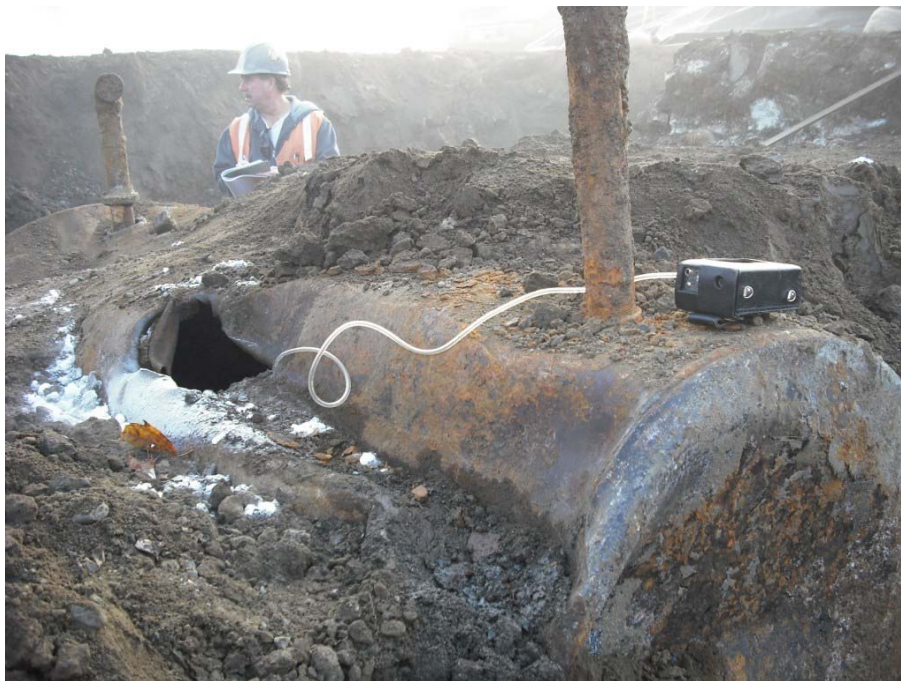
View of LEL meter taking reading from Tank 1.
