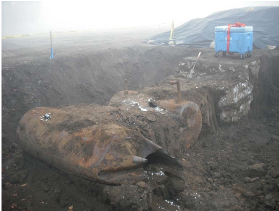
View of tanks and concrete vault facing northwest. Soil stockpile in background.
