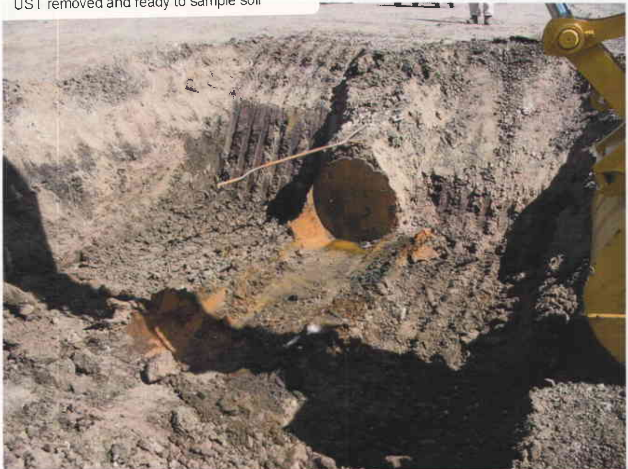
The Green on Park Place Martinelli & Arnold Road Dublin CA 94568 RWeston 10-2-08 UST removed and ready to sample soil
