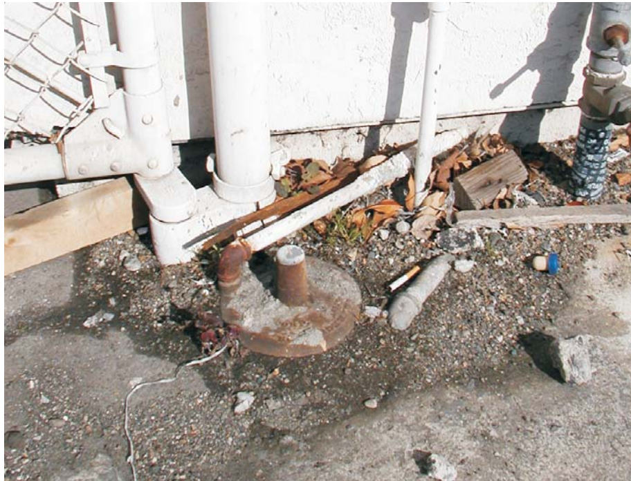
18. Possible former vent at the west side of the subject site, northwest of Building C.
