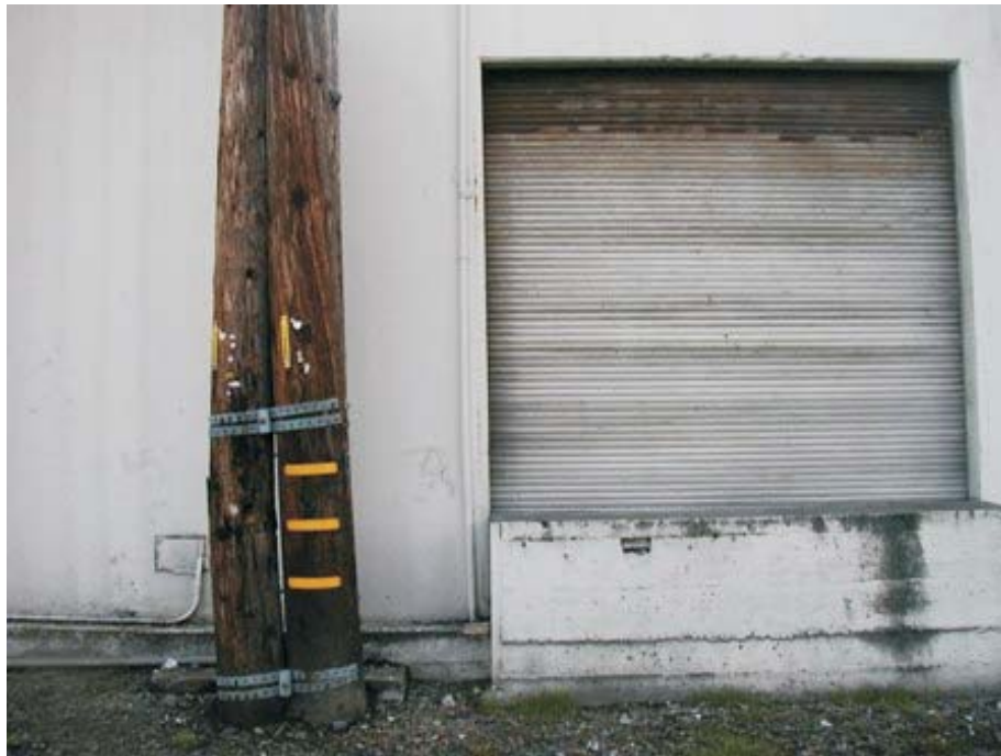
12. Bottom of the vent pipe at the east side of Building B.
