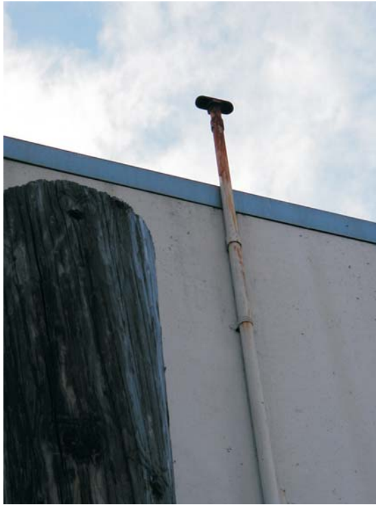
11. View of the top of a vent pipe at the east side of Building B.
