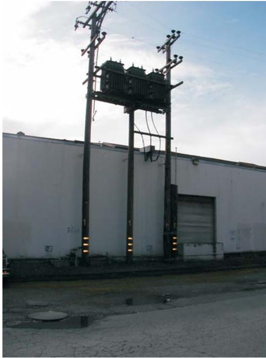
9. East side of Building B, with a view of transformers and a vent pipe.
