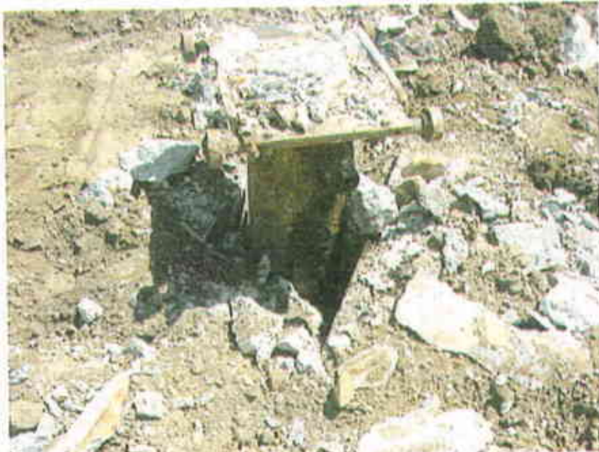
Photograph 3. Moveable hydraulic lift in concrete lined trench.
