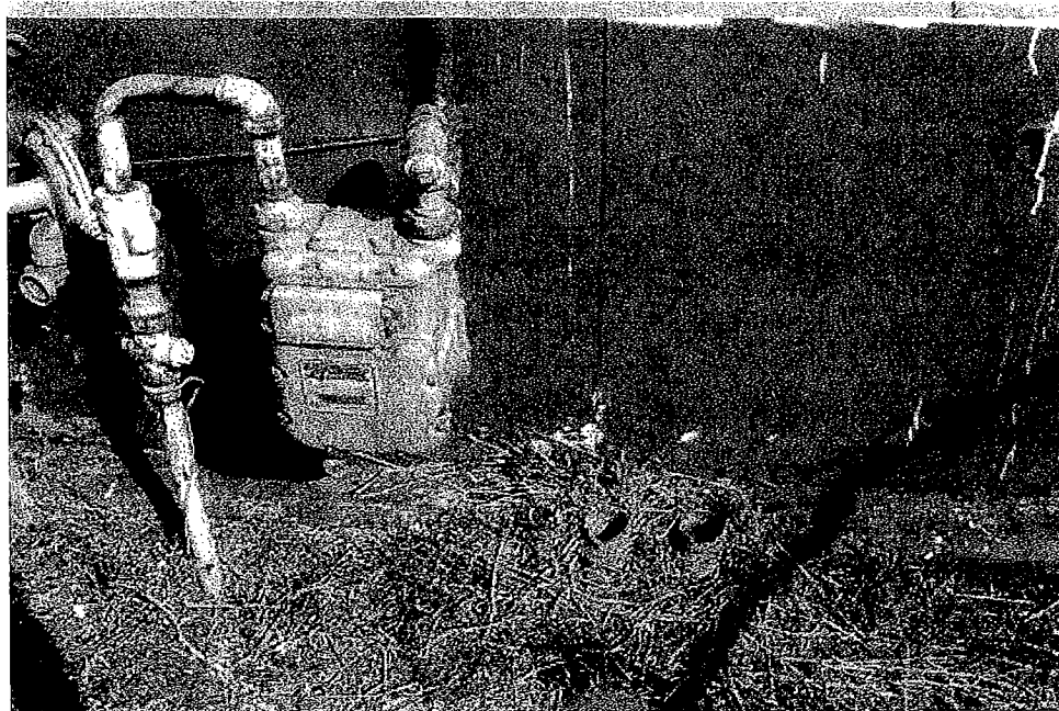
Photo 6 - View looking at the suspect vent pipes to the west of the main subject property building
