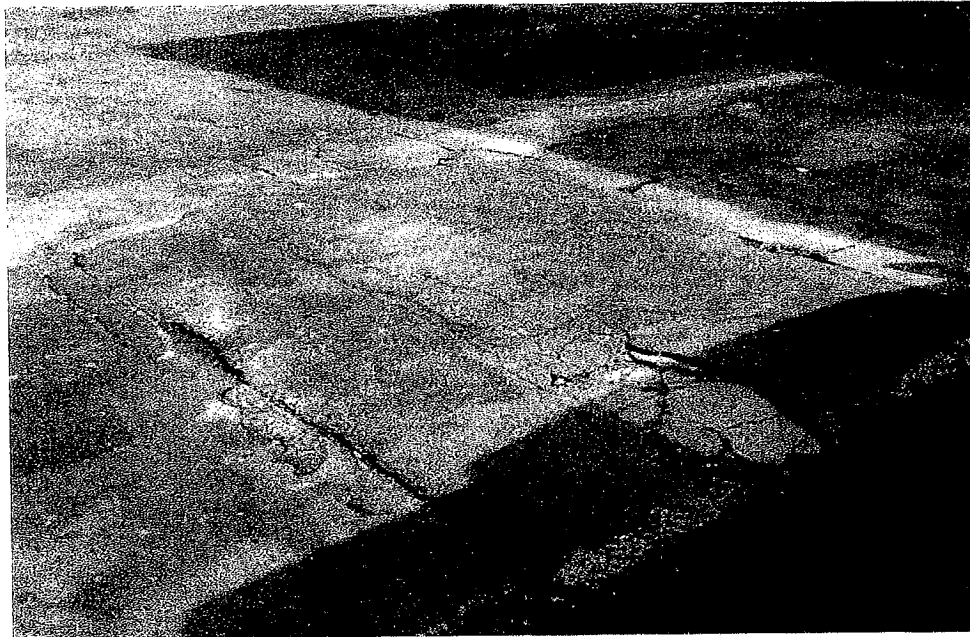
Photo 8 - View looking at the approximate location of the former canopy and suspect former underground storage tank (UST) locations on the northeastern portion of the subject property.
