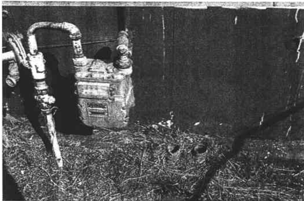
Photo 6 - View looking at the suspect vent pipes to the west of the main subject property building
