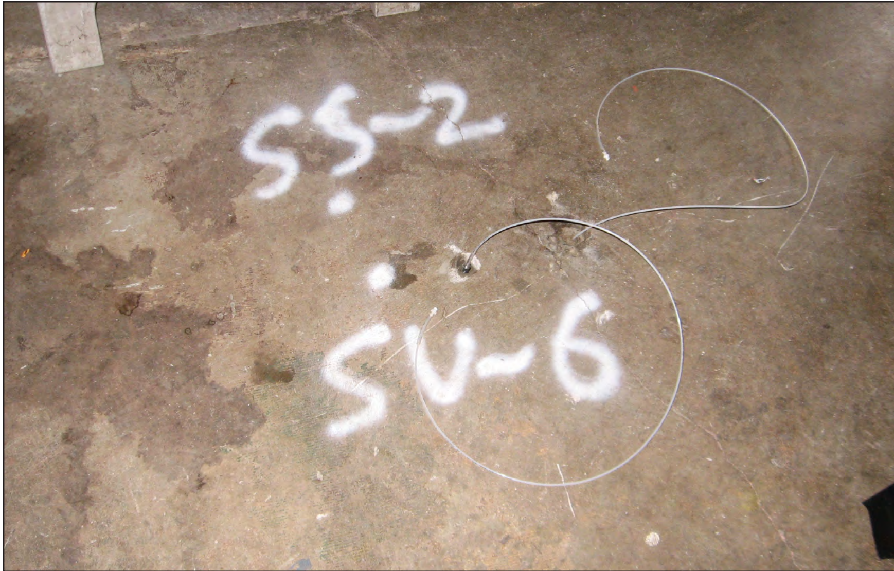
East of former dry cleaning machine location. Note floor crack.
