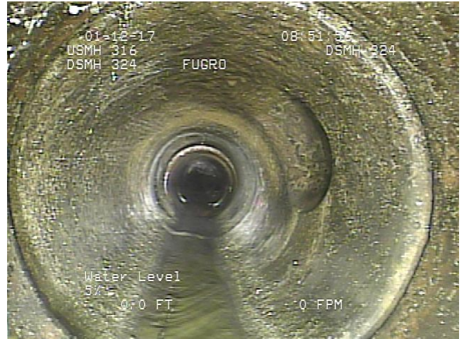
MWL - Water Level Distance: 0 Severity: None
