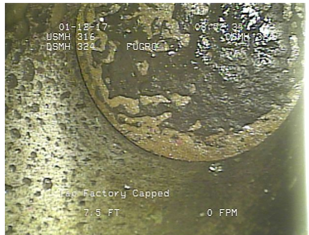
TFC - Tap Factory Capped Distance: 7.5 Position: 3 Severity: None Size: 4
