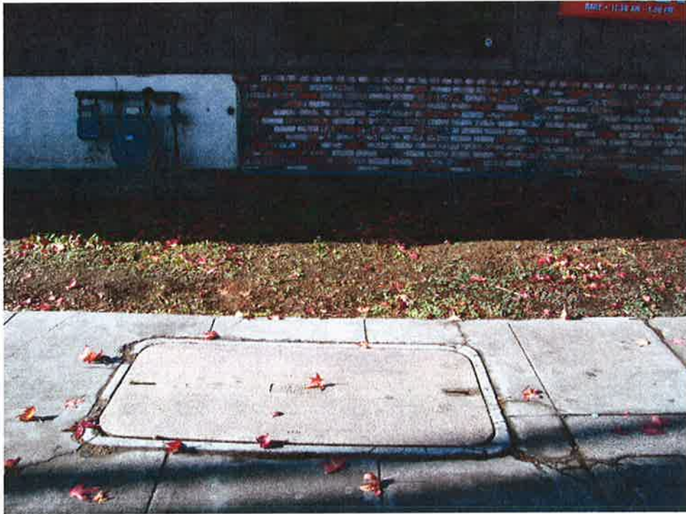
Vaults V2 (Pacbell) and V3 (Gas Meter)
