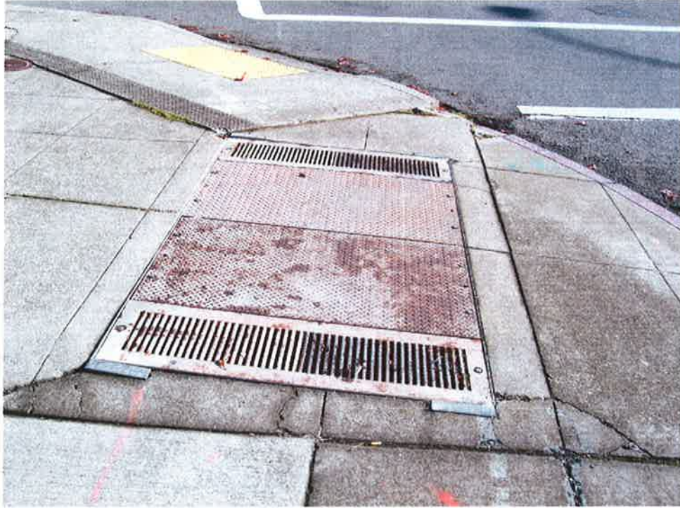
Vault V18 (Electric – Transformer HIGH VOLTAGE)
