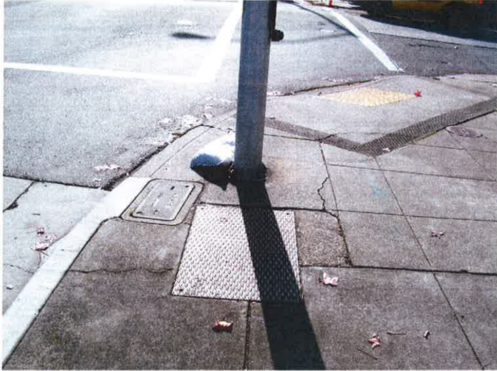
Vaults V14 (Electric –High Voltage), V15 (Traffic), and V16 (Signal)
