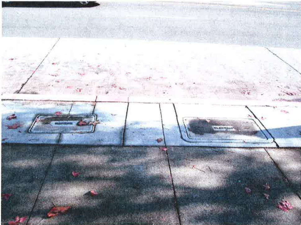
Vaults V9 and V10 (Electric – Street Light)
