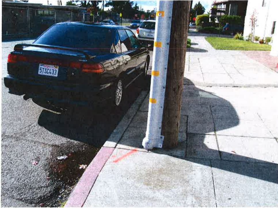
Vault V20 (Electric – Overhead Transfer to Subsurface)
