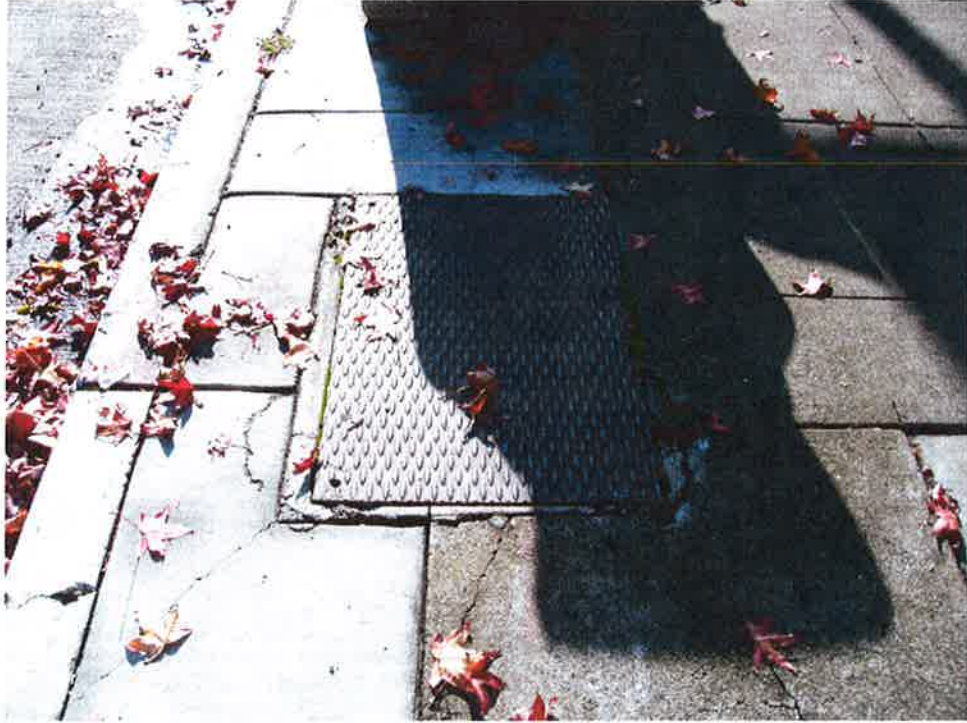
Vault V4 (Electric – High Voltage)
