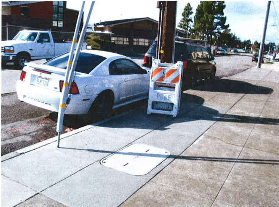
Vault V19 (Electric – High Voltage)
