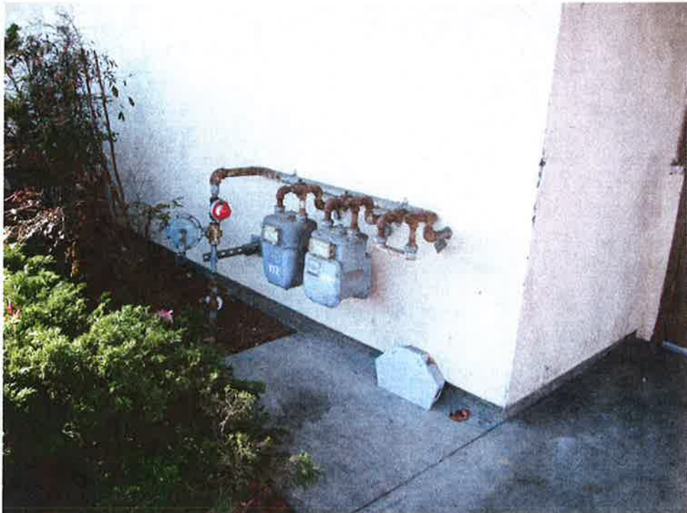
Vault V5 (Gas Meter)
