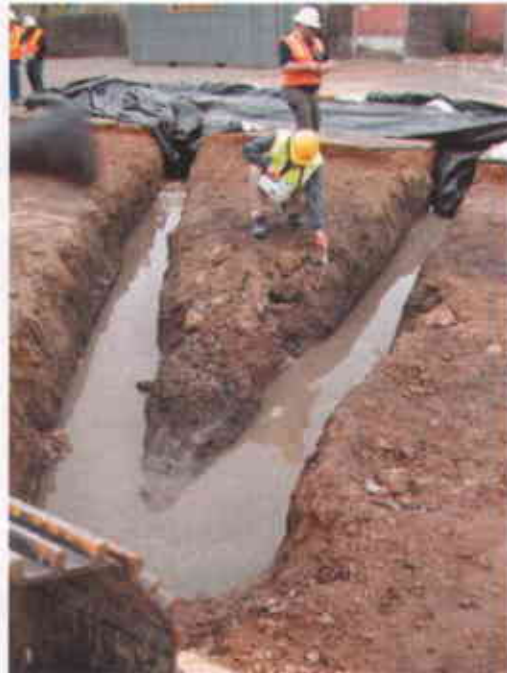
Accumulated rainwater drained into trenches; LEL monitoring near exposed soil surface (Facing north)
