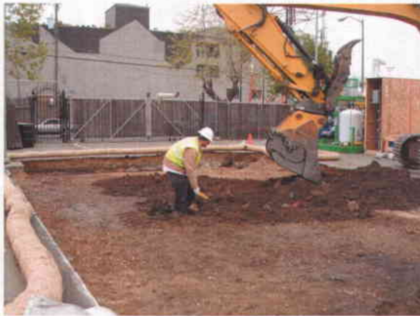
Photo #8 - Potholing a location further east within the pad footprint; since soil at this location appeared to be uncontaminated this location was defined as the “benchmark” and the eastern limit of soil excavation (Facing east; 4/25/2007)
