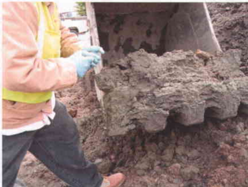
Photo #17 - Collection of confirmation soil samples in 6" X 1.5" stainless steel tubes from the materials brought to the surface in the excavator bucket (4/25/2007)
