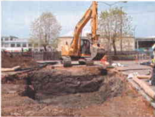
Size/shape/depth of excavation before being instructed by the City Inspector to increase the depth of excavation (Facing northwest)
