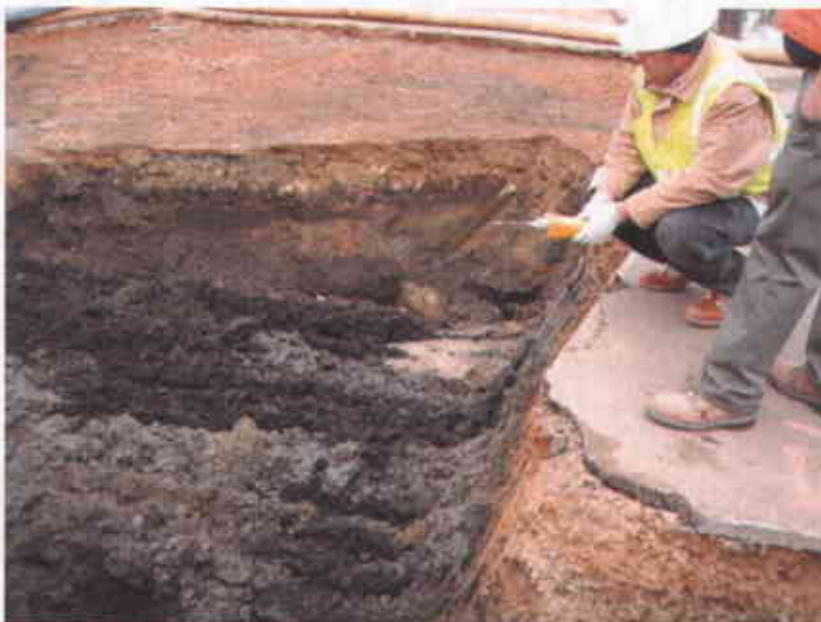
PID monitoring near the excavation surface; note the black color of the odor-causing soil (Facing east)
