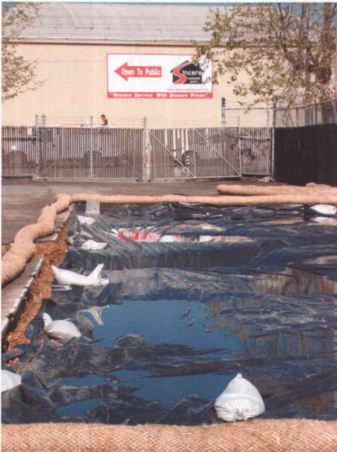
Photo #2 – Prior to the start of the removal action contractor had left site covered with plastic sheeting – note the accumulated rainwater (Looking west; 4/20/2007)
