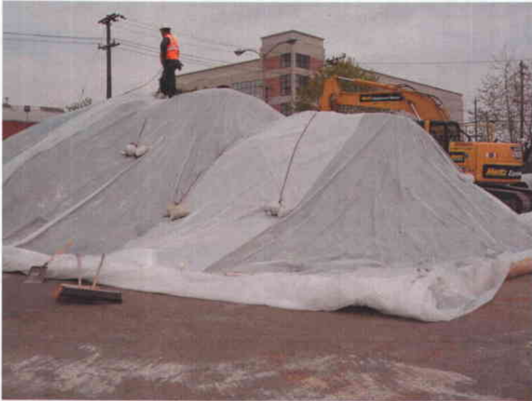
Photo #14 - Stockpile, covered with Visqueen sheets, weighed down with sandbags and bordered with straw wattles (Facing East; 4/25/2007)
