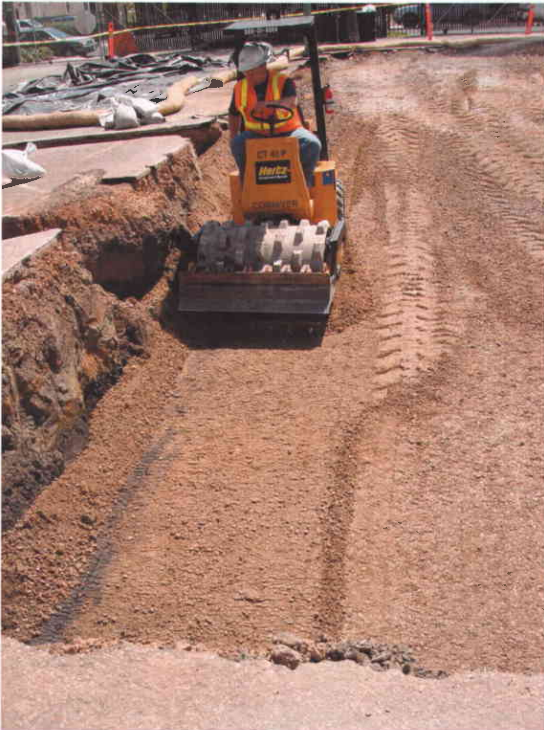
Photo #21 – Backfilling operations: Initial use of a one-ton John Deere CP-40 sheep foot compactor for backfill compaction (Facing east; 4/26/2007)
