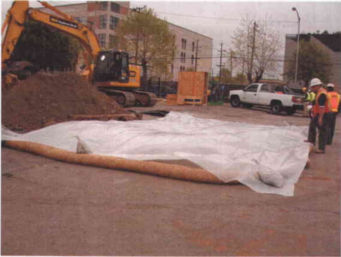
Photo #13 - Additional Visqueen® sheet being placed on the ground to expand the existing stockpile area (Facing east; 4/25/2007)
