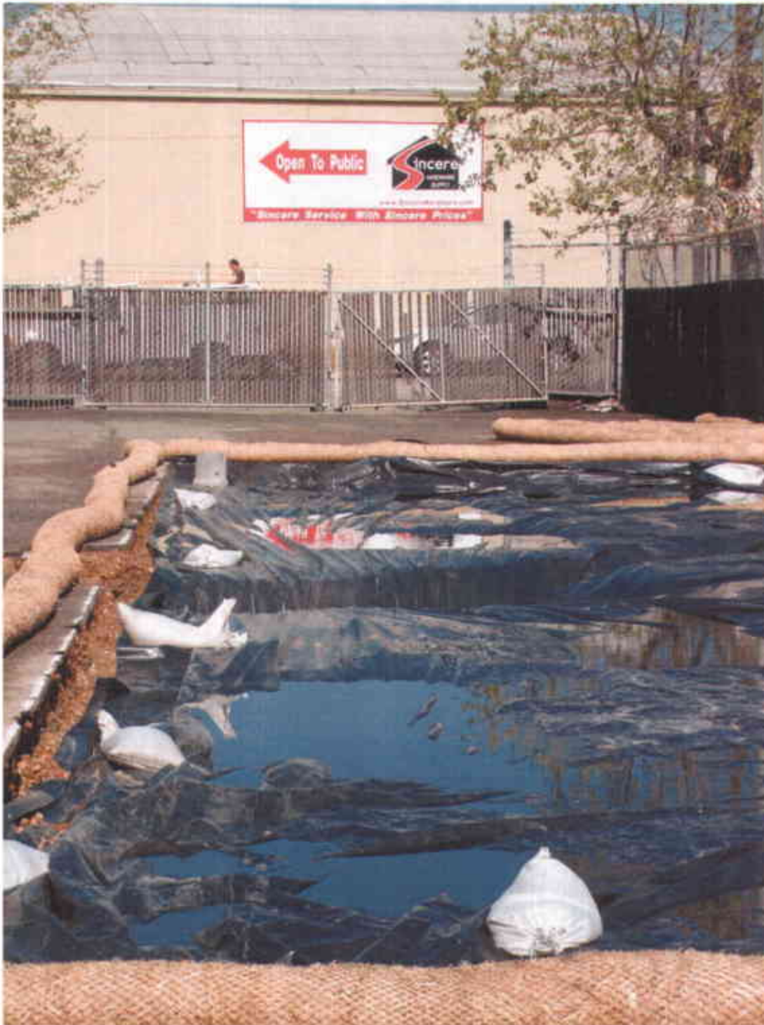
Photo #2 (4/20/2007)– A view of the area being excavated for building pad construction, note the accumulated rainwater on the plastic sheeting covering the equipment pad excavation.
