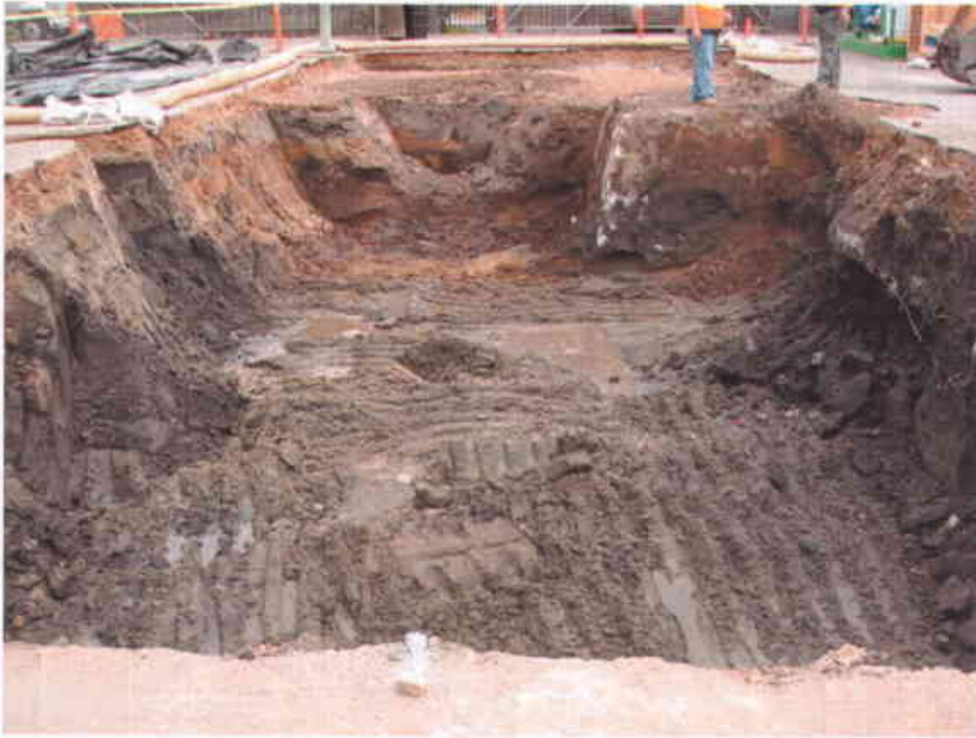
Photo #9 - View of final excavation (~ 7 ft deep) after confirmation sampling – note the old concrete foundation under man's feet (Looking east toward Brush Street; 4/25/2007)
