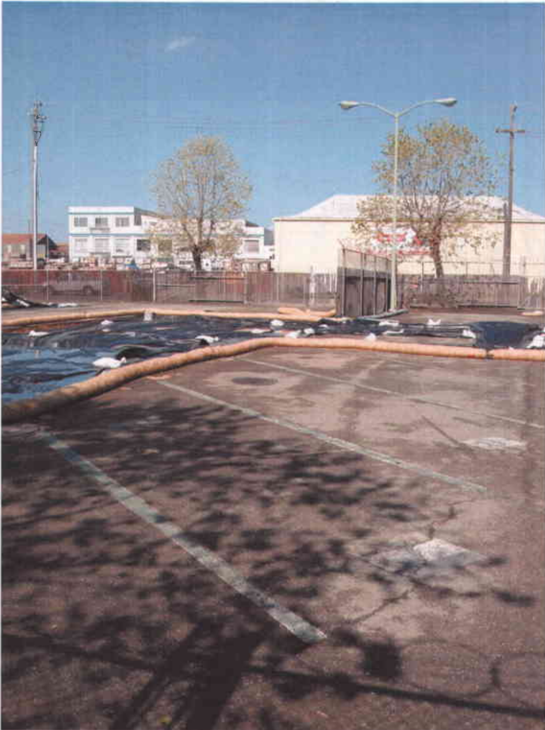
Photo #3 (4/20/2007) – Another view of the building pad excavation area. Equipment pad excavation is on the left side and the dispenser excavation is on the far right side of the photograph.
