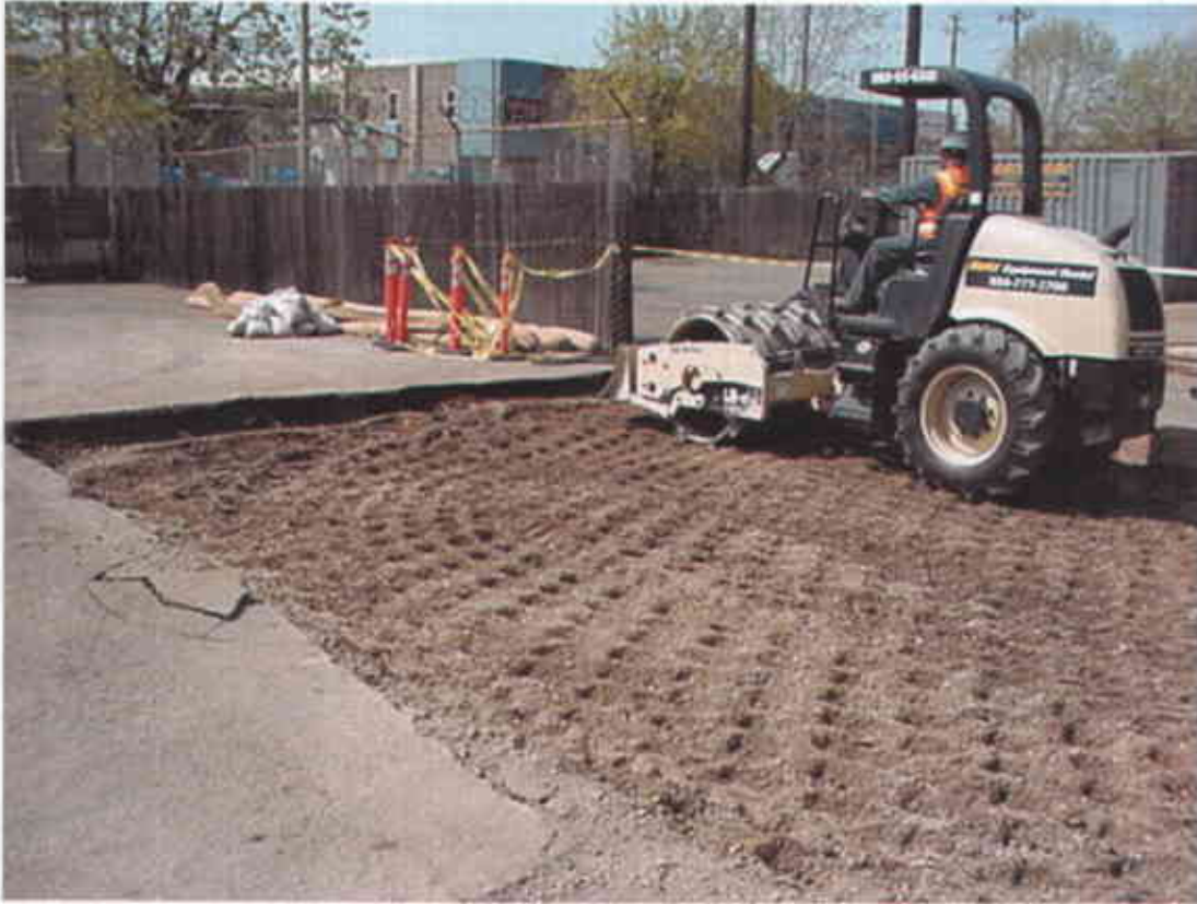
Photo #23 – Backfilling operations: utilizing a 5-ton Ingersoll-Rand SD-45 sheep foot compactor (Facing north; 4/27/2007)
