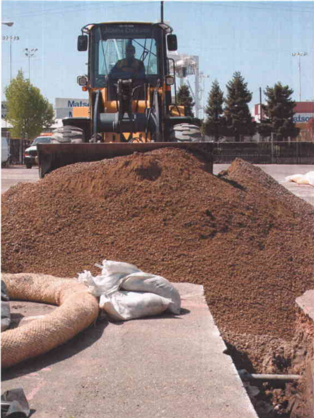
Photo #19 – Backfilling operations: John Deere 544 loader pushing backfill material into the excavation (4/26/2007)
