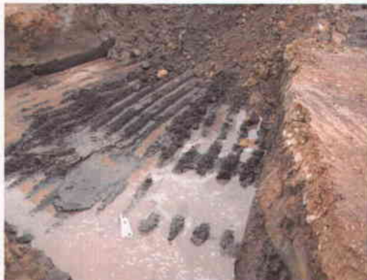
Rainwater drained into the excavation
