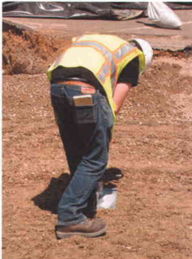
Photo #22 – Backfilling operations: Field compaction tests being conducted with a Troxler Nuclear Gauge (4/26/2007)
