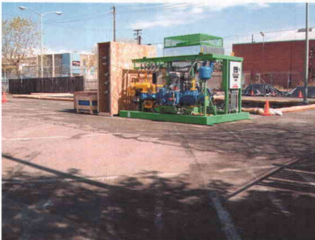
Photo #1 (4/20/2007)– One of the two CNG Compressor Units for the Fueling Station. Equipment pad is located immediately behind the compressor unit. View towards the northwest.
