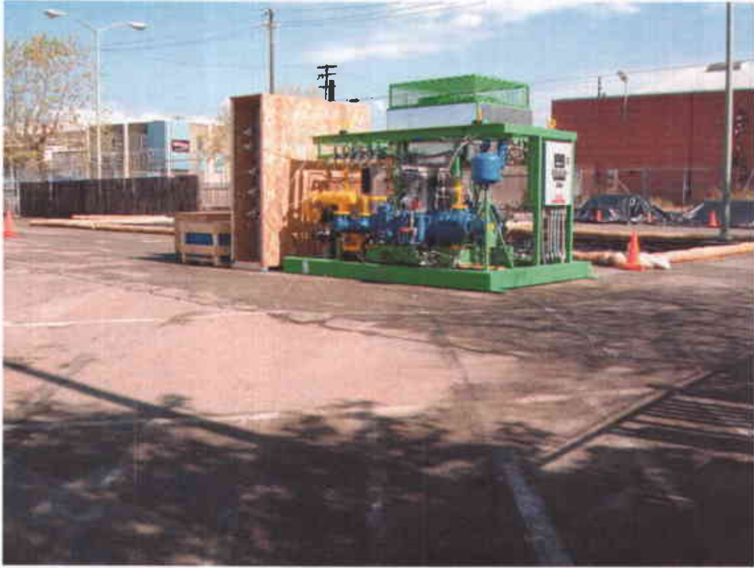
Photo #1 – One of the two CNG compressor units for the fueling station (Facing north; 4/20/2007)
