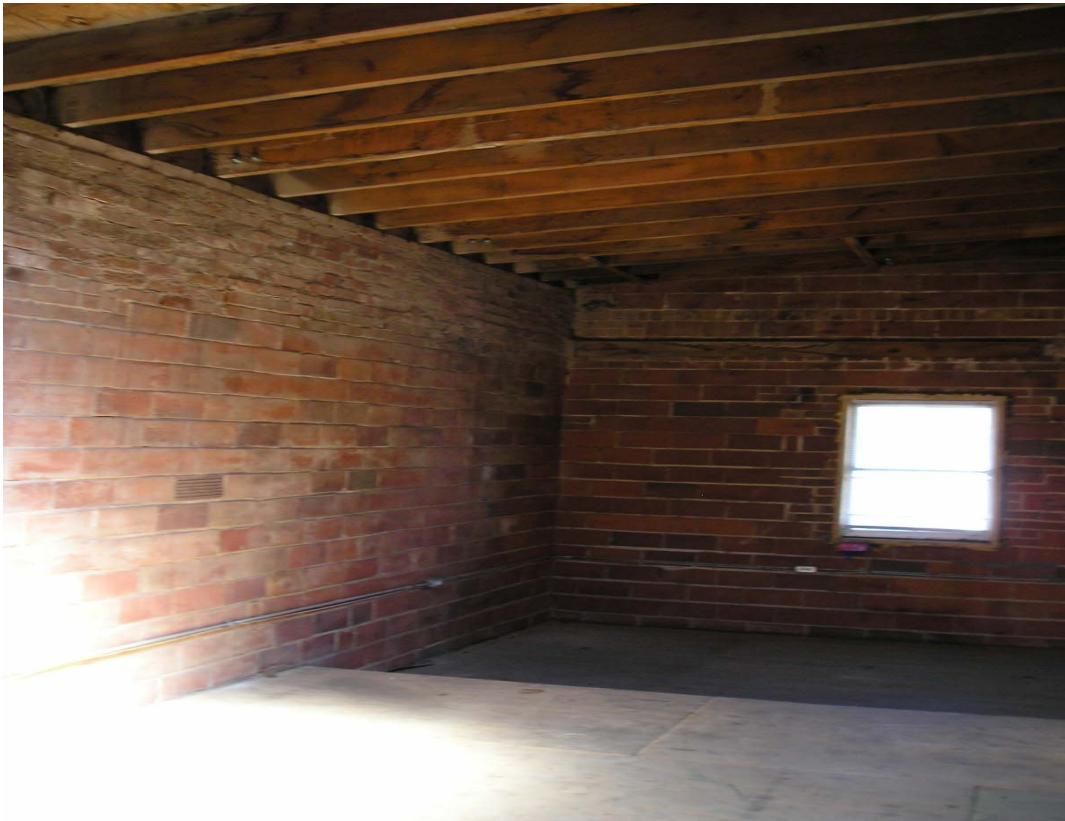
Photograph 8: Interior of 3005 E. 12th Street. Note elevated slab detail along north side of building.
