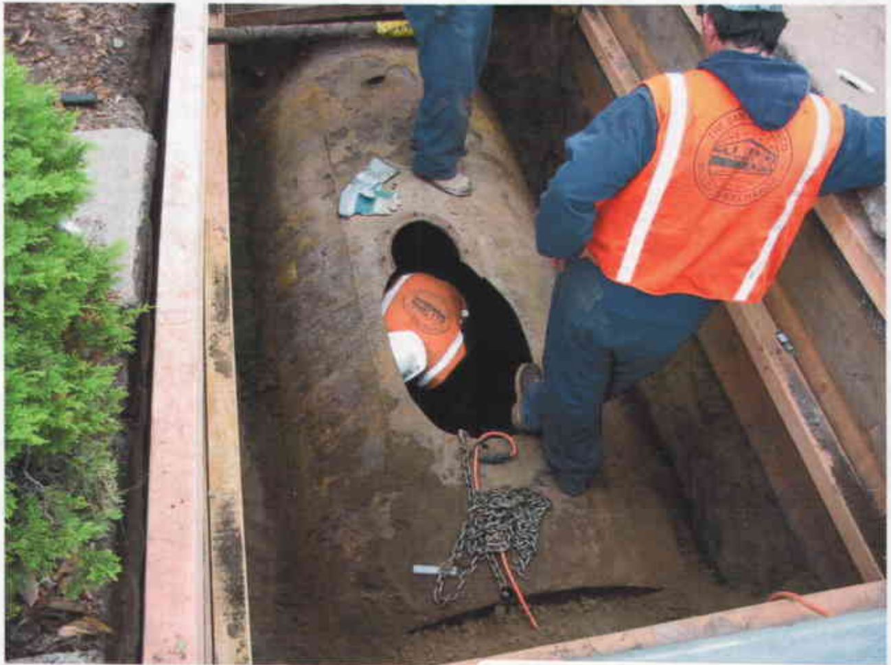
Residential apartment building 757 Santa Clara Avenue Alameda CA 94501 RWeston October 16, 2007 tank previously cleaned, tank cut into two pieces
