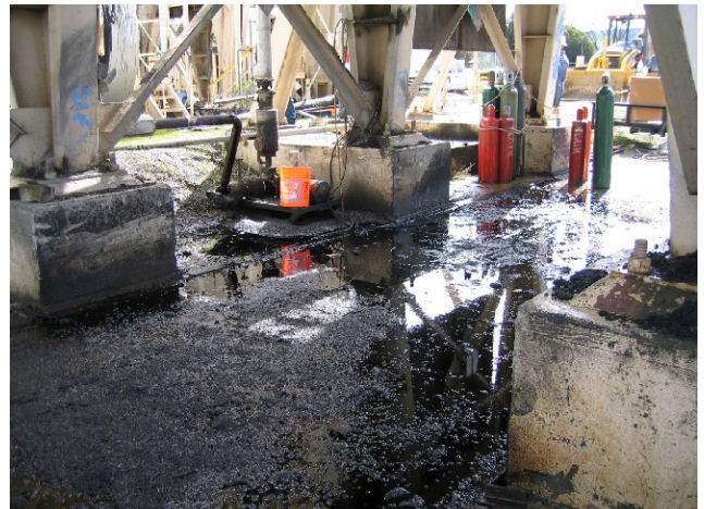
4. Oil spill beneath loading silos at asphalt batch plant, caused by demolition operations. Crew later applied absorbent to the spill.
