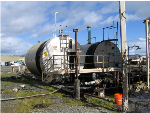
3. Above ground paving oil tanks at asphalt batch plant, southwest corner of main improved parcel. Plant is currently being demolished.
