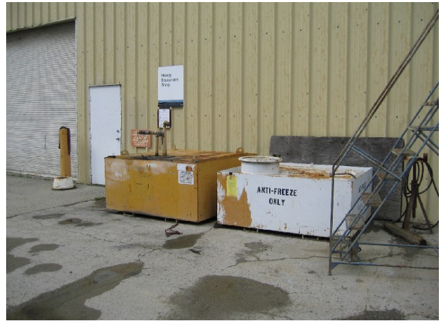
2. Waste oil (left) and waste antifreeze aboveground storage tanks, south side of heavy equipment shop building.
