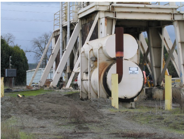
5. Integral oil tank for column heating apparatus, asphalt batch plant. Unit is scheduled for demolition.
