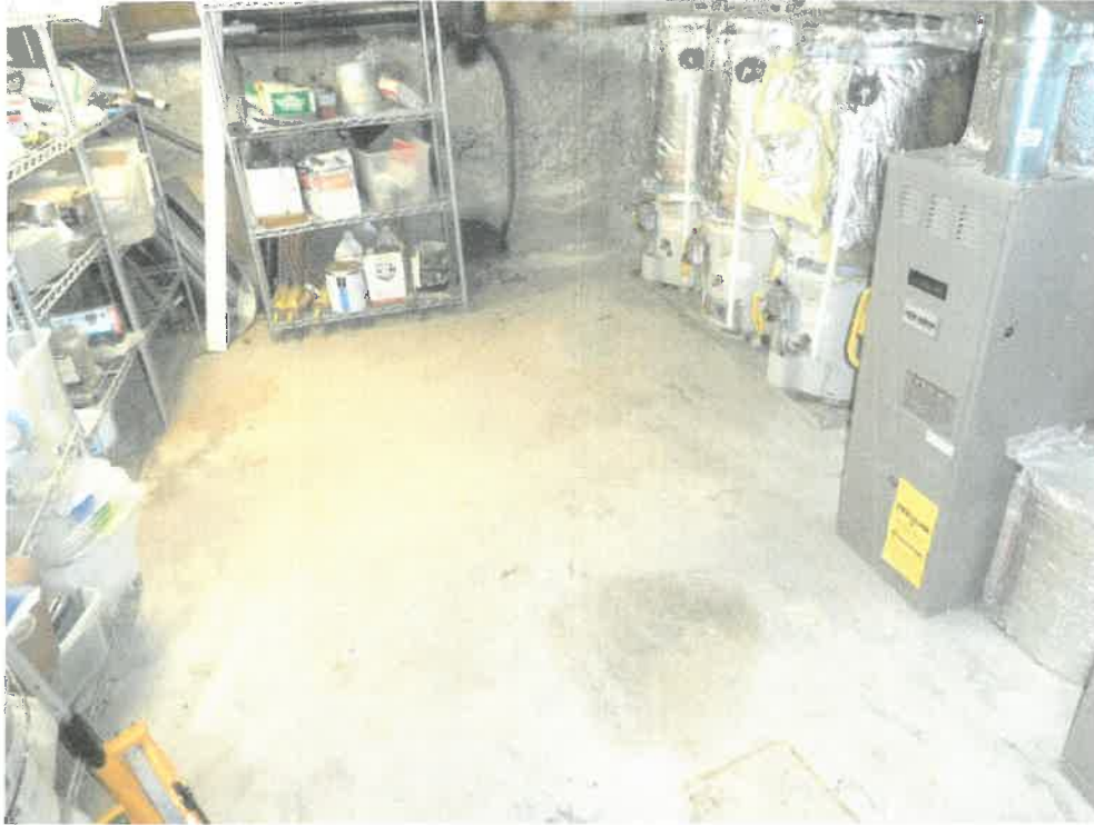
Photo 1 – Gas furnace and water heating in the basement in the back
