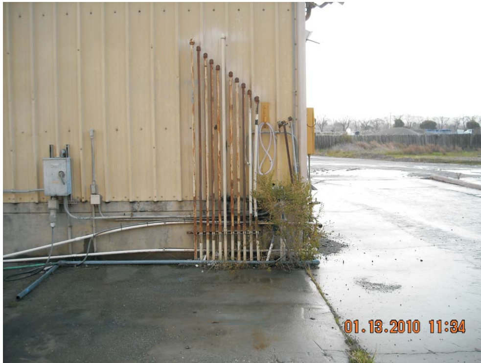
10 - 1-INCH DIAMETER PIPES AT THE LUBE SHOP
