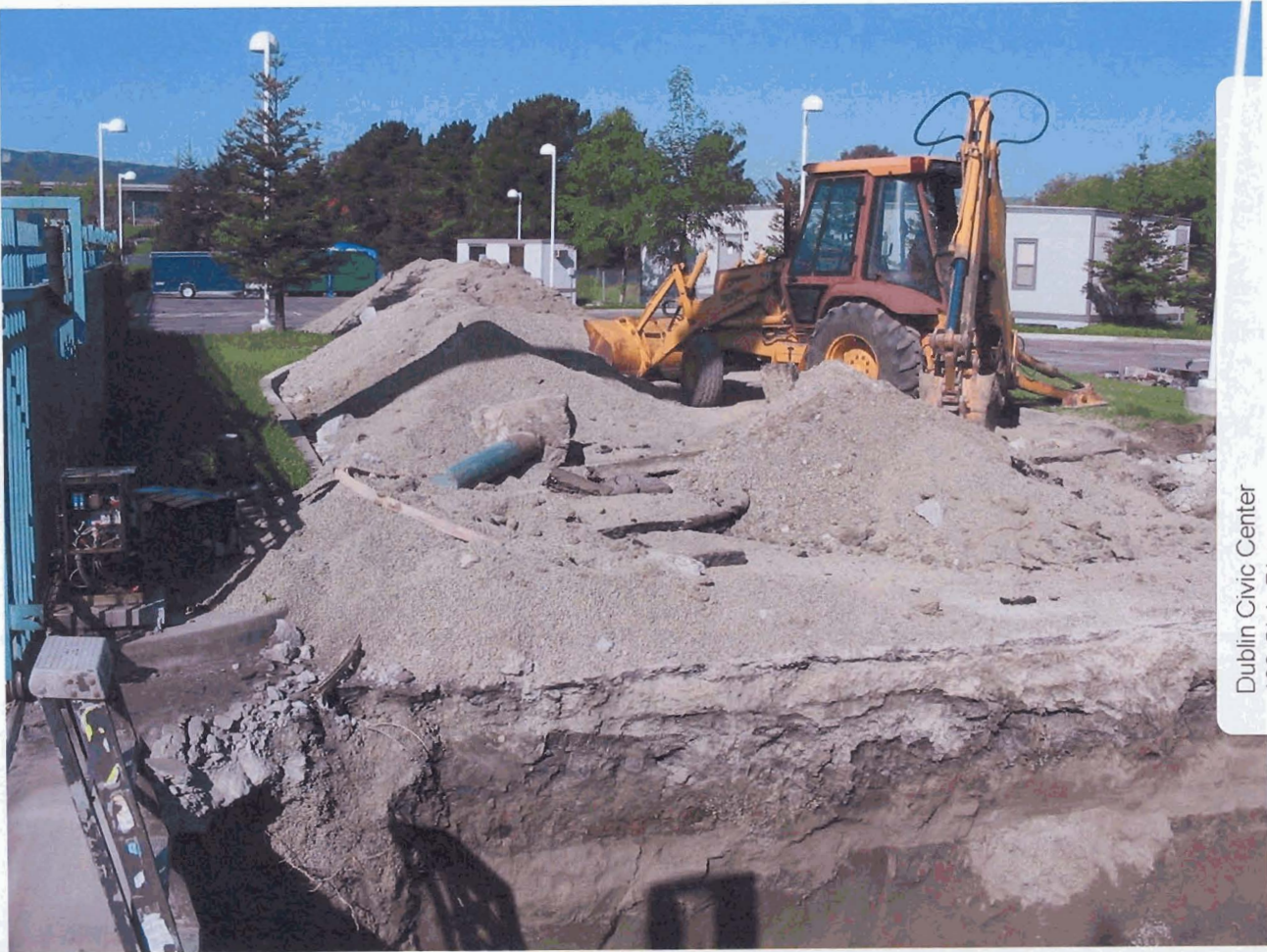
Dublin Civic Center 100 Civic Plaza Dublin, CA 94568 RWeston 5-1-2006 10K gasoline tank removal, UDC and piping to the tank, in-situ
