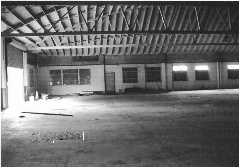
Photograph 8 - View of the interior of the smaller concrete tilt-up warehouse looking east.
