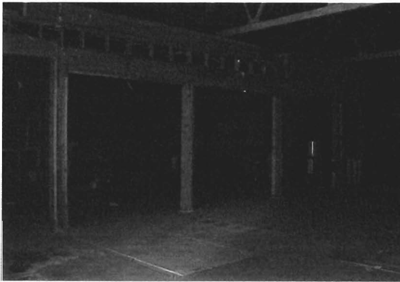
Photograph 11 - View of the wooden frame of the old office located in the larger concrete tilt-up warehouse on the Property.
