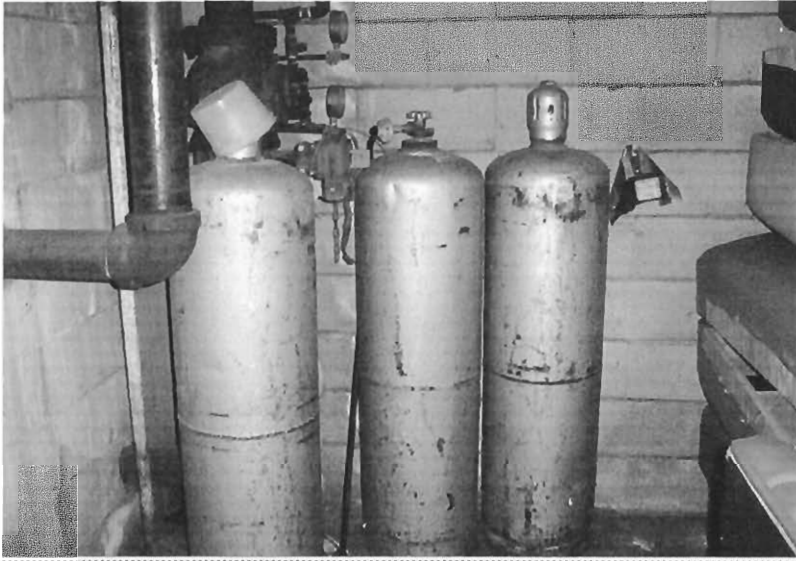
Photograph 7 - View of the propane cylinders in the cinder block warehouse on the Property.
