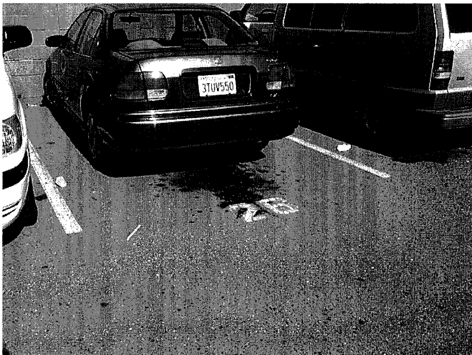
Photograph 2: View of surficial staining in the parking lot.
