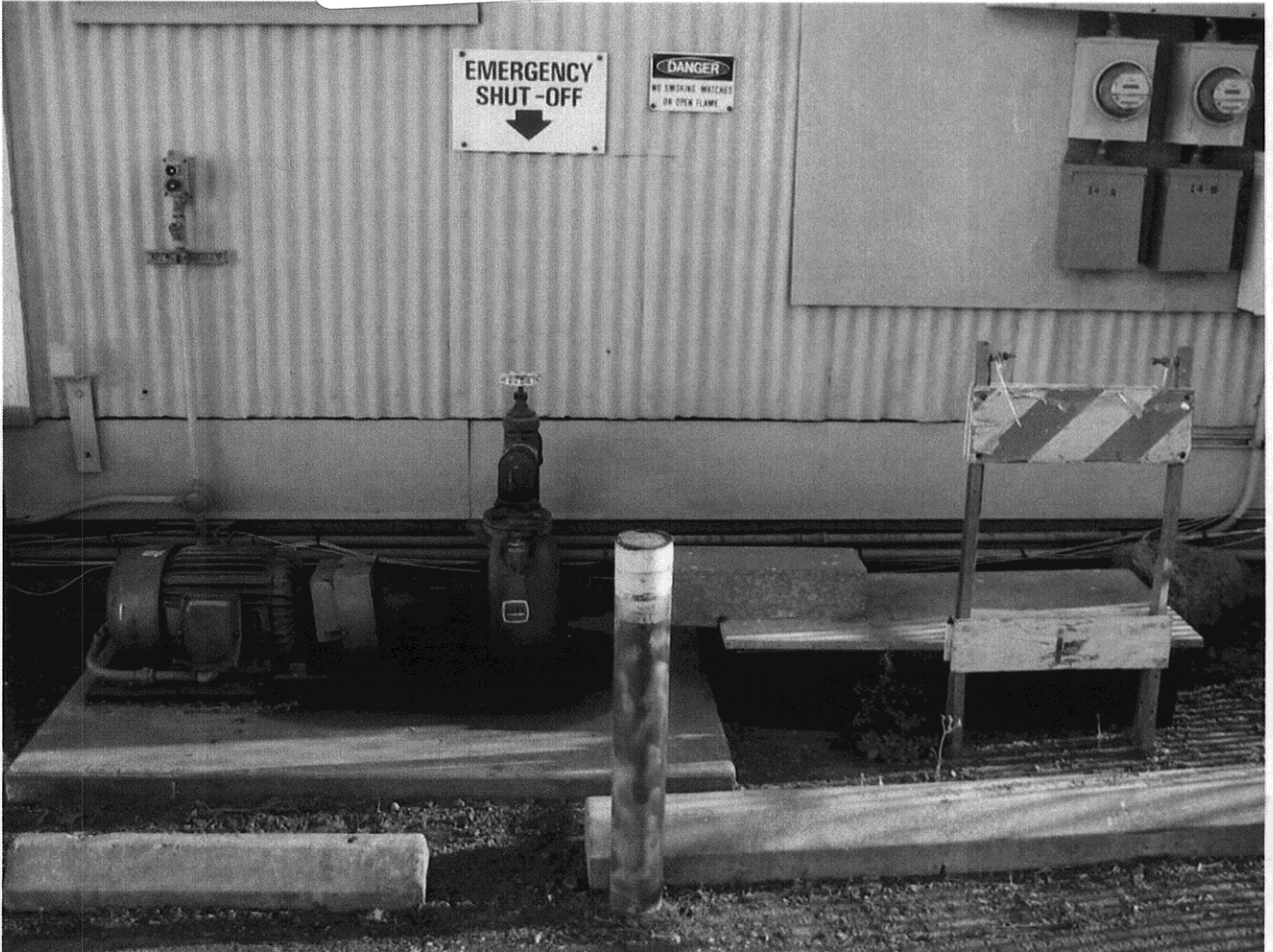
Grand Harbor Fuel Dock 2099 Grand Street Alameda CA 94501 High flow piping pump & sec cont basin RWeston
